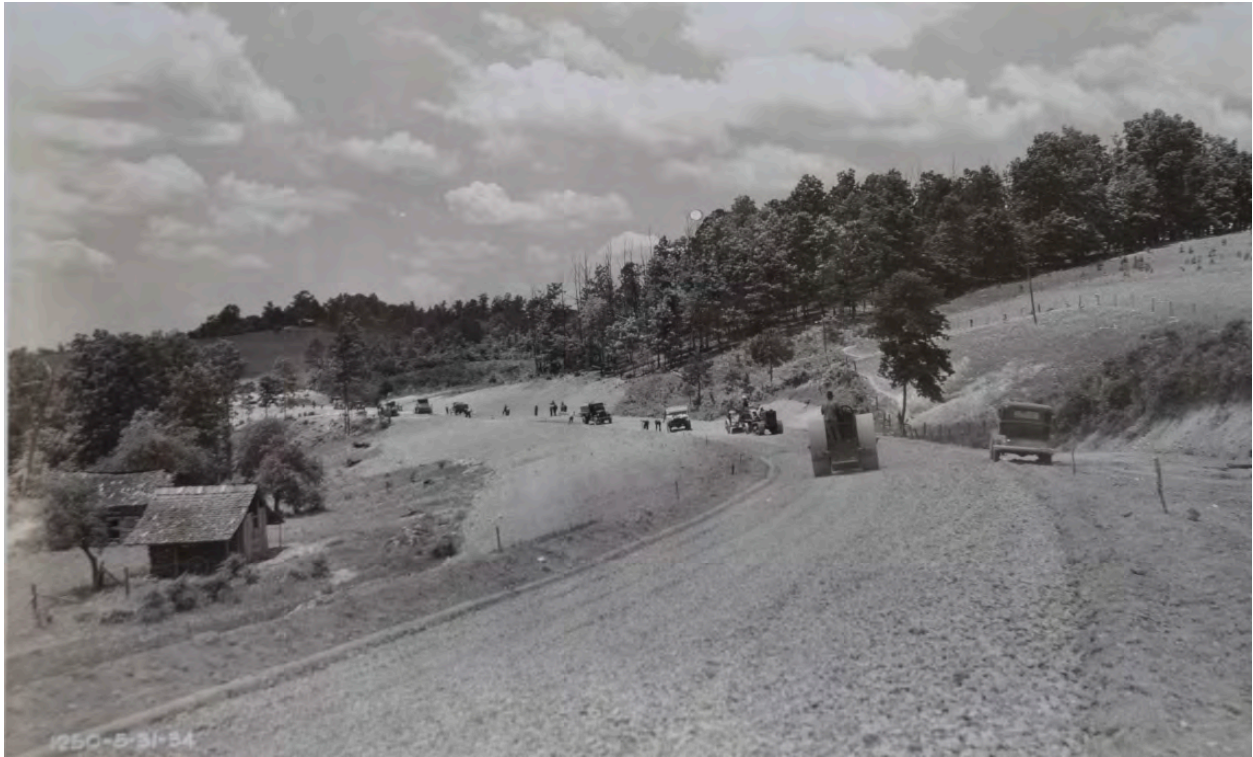
Norris Freeway grading was underway in 1934 south of the town of Coal Creek.
