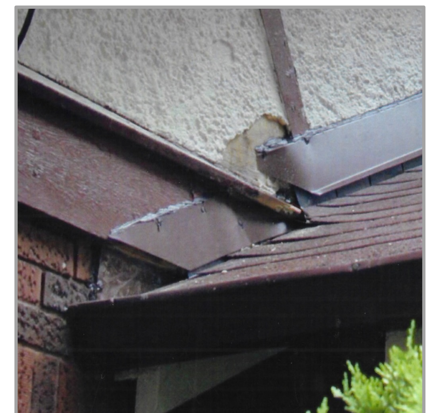
Water damage from roof or plumbing leaks can cause indoor problems like mold.
