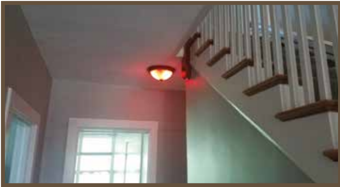
For a homeowner who is deaf, alternating ceiling lights throughout the house can alert inhabitants to many different kinds of important information.
