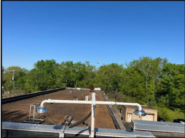
Figure 3-4: East Health Center (WEST)
