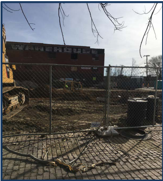
This photograph shows remedial and redevelopment activities underway on the property in 2017.
