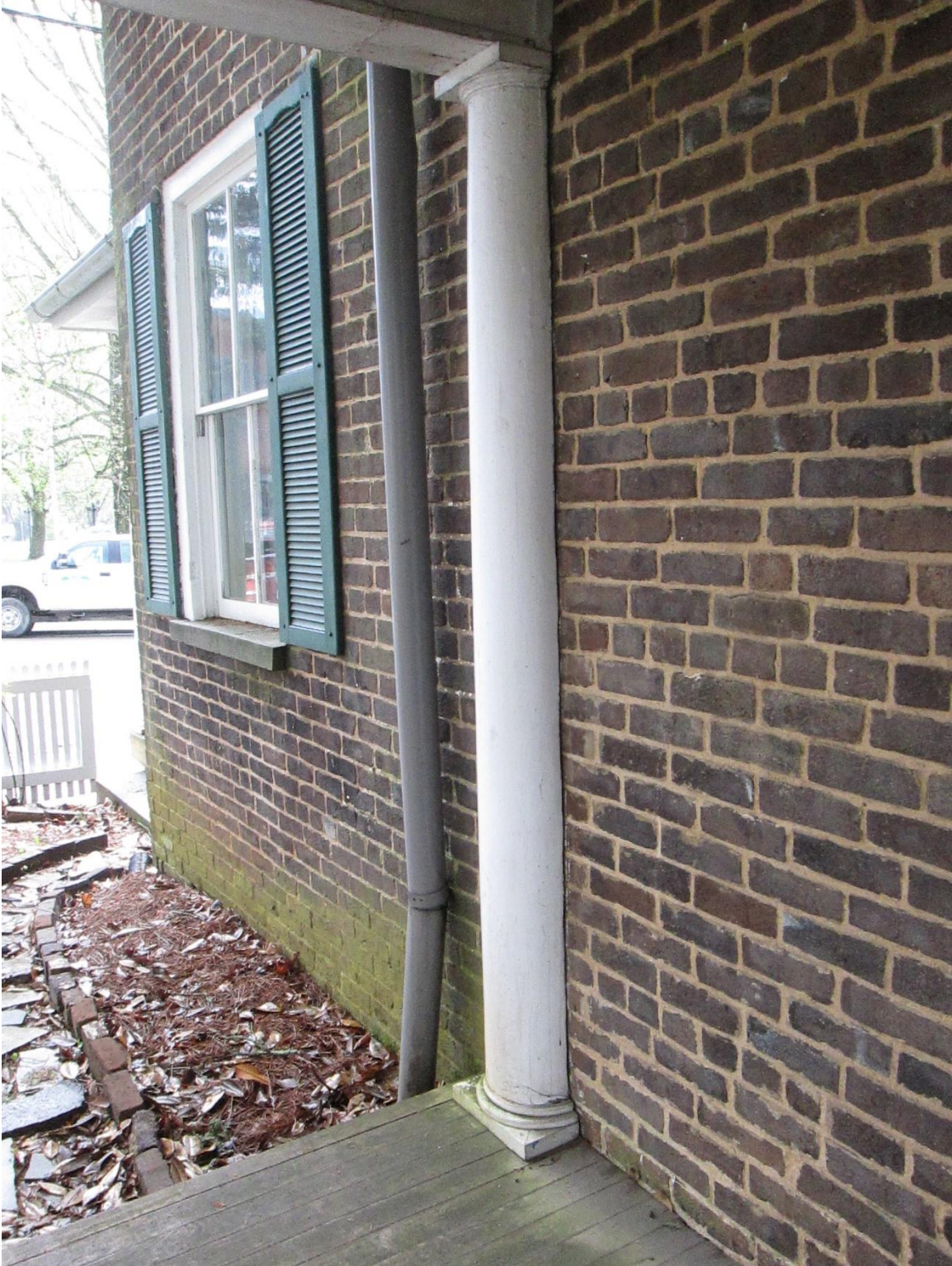
Photograph 6. Example a pilaster along the north elevation of the Nance Building in fair condition.
