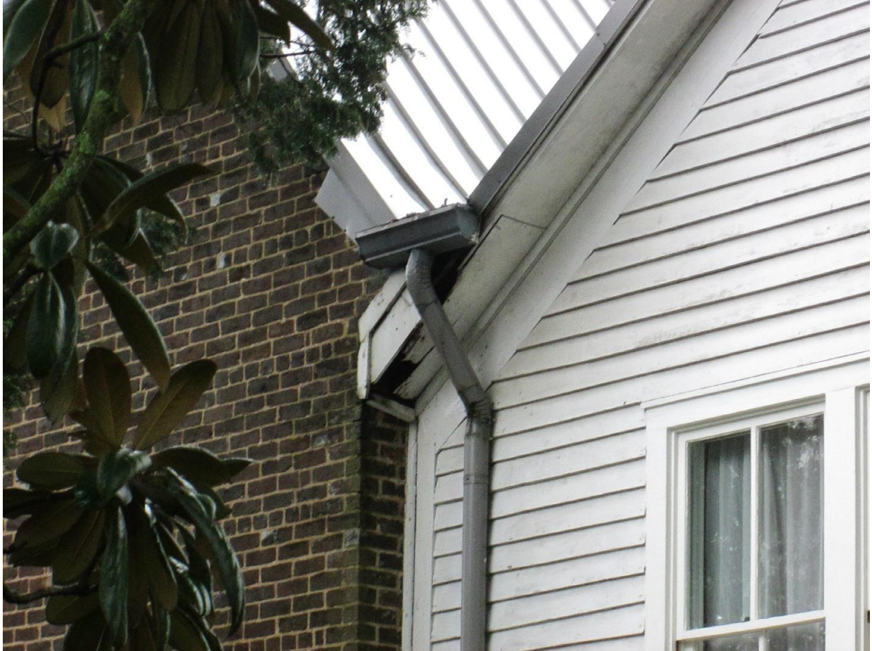
Photograph 10. Detail view of soffit along the north elevation gable of the Nance Building showing substantial deterioration.
