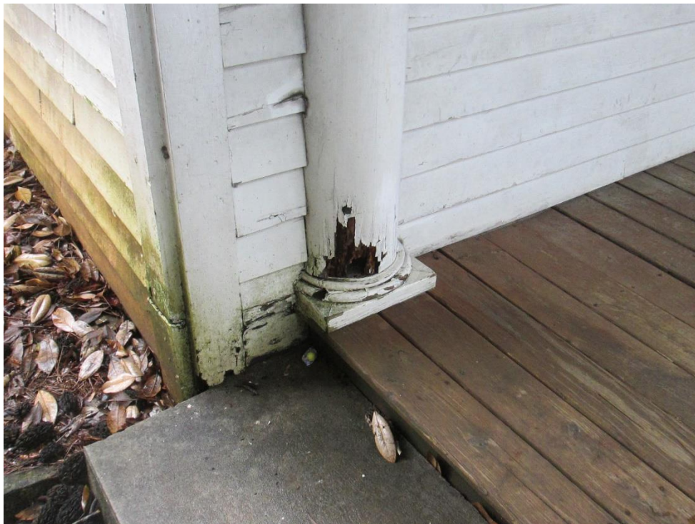
Photograph 3. Example of substantial deterioration of a pilaster along the west elevation of the Nance Building.
