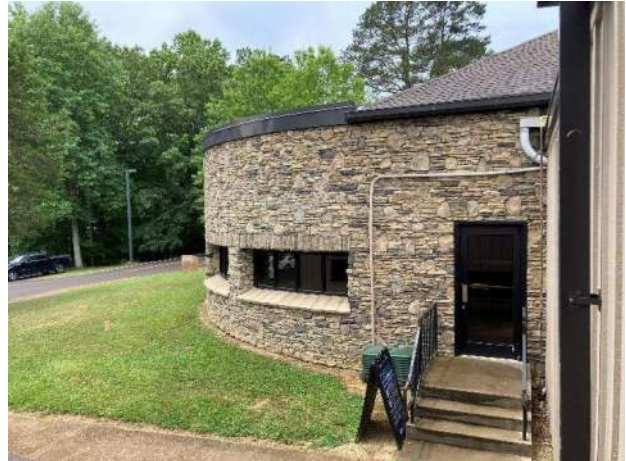
21) Lodge Exterior – View of exterior stone veneer, which appears in good condition. Asphalt shingle roofing and all roof coping appeared in good condition.
