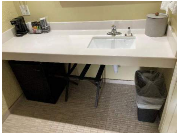
75) Guest Area – View of recently updated guest room. It was noted that all rooms are experiencing extreme condensation issues.
