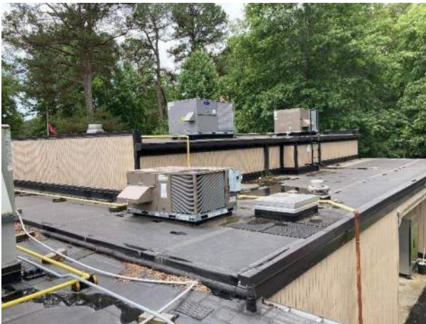
78) Roof – View of the conference area. Refer to MEP narrative for additional information.
