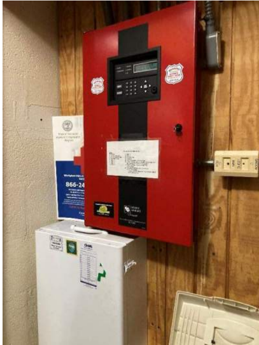
56) Back of House – Main Fire Alarm panel located behind the reception desk. Refer to MEP narrative for additional details.
