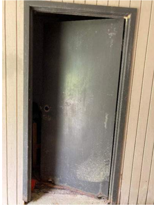
73) Guest Area – Several finishes on the lowest level show signs of water damage.
