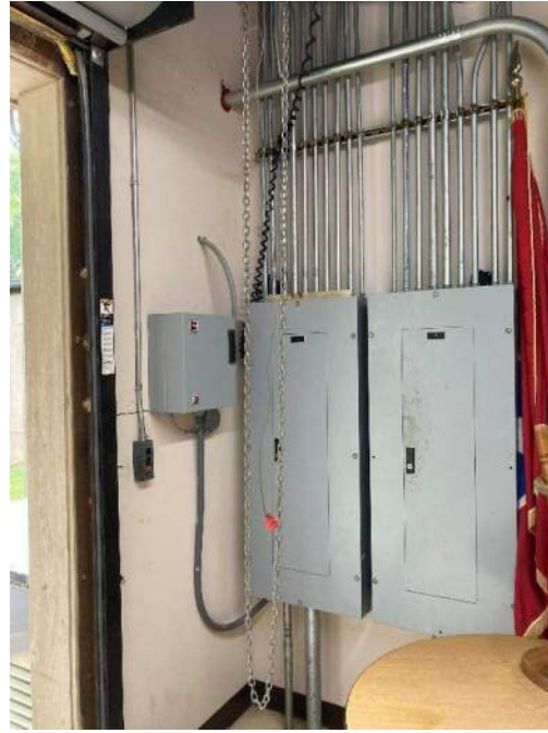
57) Back of House – Electrical panels located in the conference loading area. Refer to MEP narrative for additional details.
