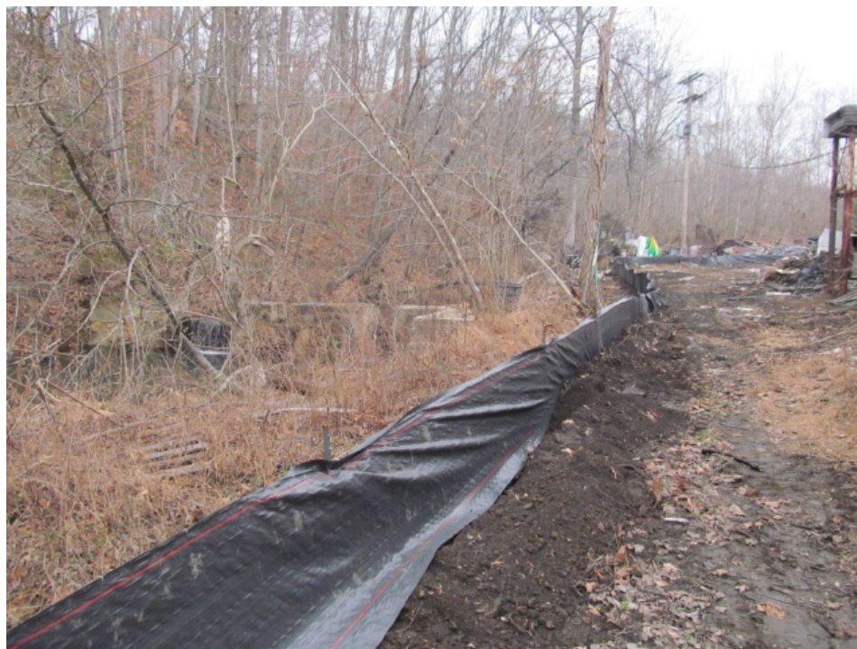
Silt fencing was installed on December 21, 2013 to keep the burned materials and soil used to extinguish the fire from entering North Fork of Mill Creek. This location is behind the main building. View is to the north-northeast. Source: EPA.
