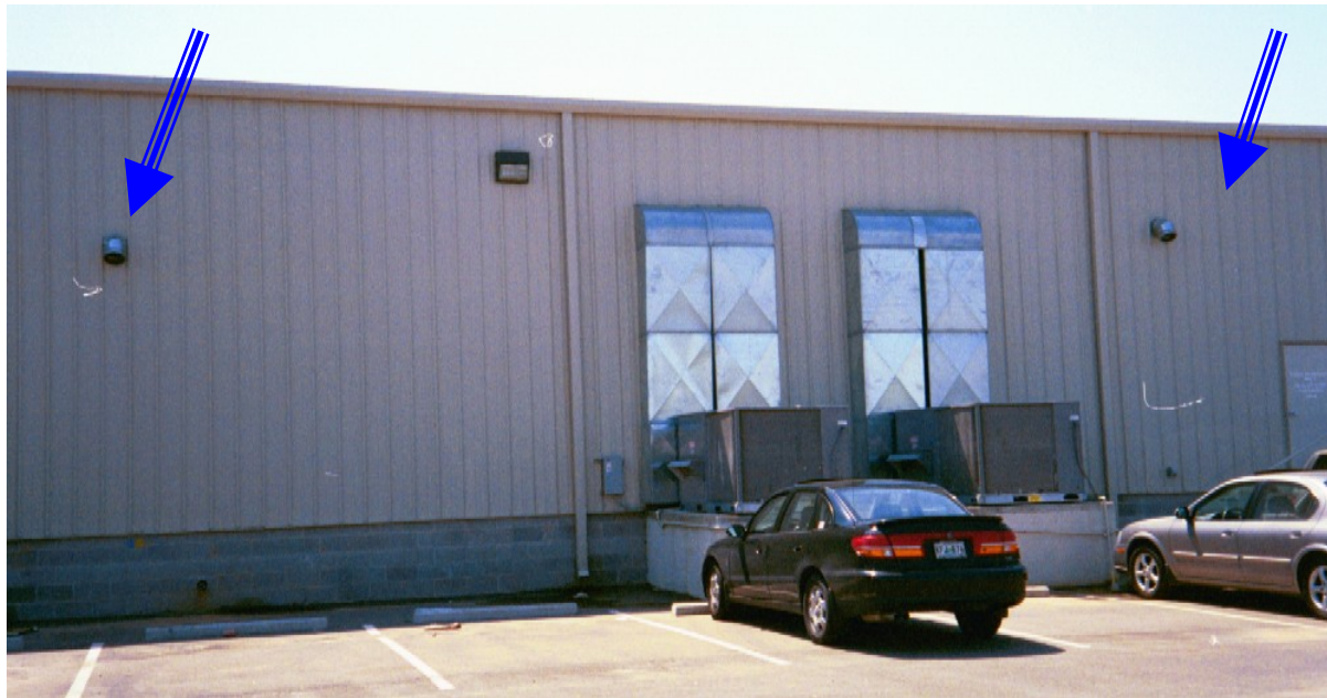
781B – Two recently installed vents to increase indoor/outdoor air exchange Jackson, Madison County, Tennessee (Photo credit: David Borowski, TDH 4/15/03)
