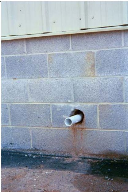
781B – One of two recently installed PVC vent pipes through solid foundation Jackson, Madison County, Tennessee (Photo credit: David Borowski, TDH 4/15/03)
