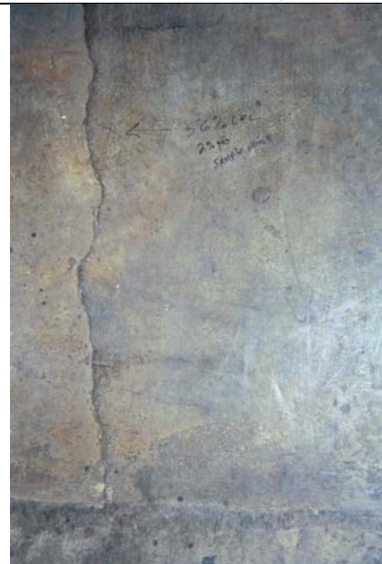
781A – Bakery store concrete floor “56% LEL 2% gas sample point” Jackson, Madison County, Tennessee (Photo credit: David Borowski, TDH 4/15/03)
