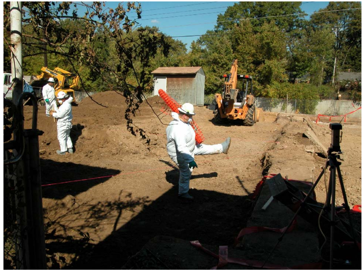
Figure 3. On-going remediation of a residential property. Two feet of soil was extracted. Orange mesh was installed before clean soil was filled and the yard's vegetative cover repaired. (photo – David M. Borowski, Oct. 26, 2005)
