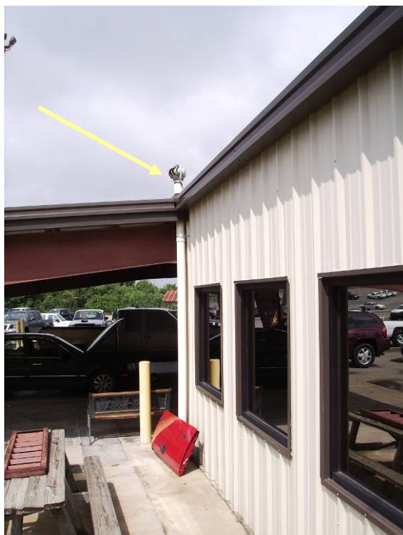
FIGURE 5. The southern side of the small graveyard building. One of two vapor vents is marked. This small building contained offices for about three employees. In the past, methane gas levels were highest within this building. A passive exhaust system was installed in December 2003 to prevent landfill gas from building up within the confined space. In December 2005, additional maintenance including caulking the floor cracks was performed to limit vapor intrusion into the building. Even with the vapor mitigation system in place, workers mentioned that unpleasant odors were often present in mornings. The building has both heating and cooling systems for indoor air climate control and ventilation.
