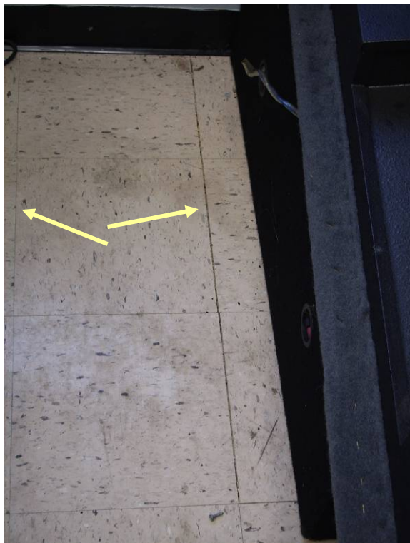
FIGURE 6. Floor tiles near the northeastern corner of the graveyard building. A previous floor crack in this area had been described as having a noticeable movement of “air” coming up through the crack. The floor had been reported to have been redone in the past few years. Even with the passive vapor mitigation system operating, widening of the floor tiles has been noticed where a past floor crack had been located. Compare the tight seem of the tiles on the left to the small gap between the tiles on the right.
