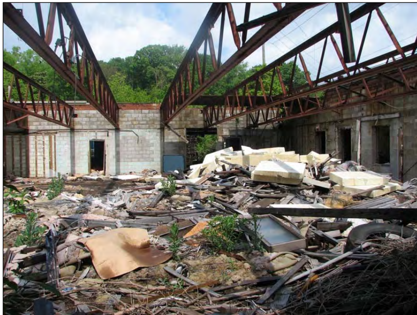
Figure 10. Scattered debris inside the former Anchor Glass Corporation office building on Tax Parcel 167C H 002 of the Oakland Avenue and 45 th Street (Alton Park Area 3) site, Chattanooga, Hamilton County, TN. (Photo credit: Sarah Stuart Chewning and Sabrina Novak, Chattanooga-Hamilton County Health Department – 5/7/09)
