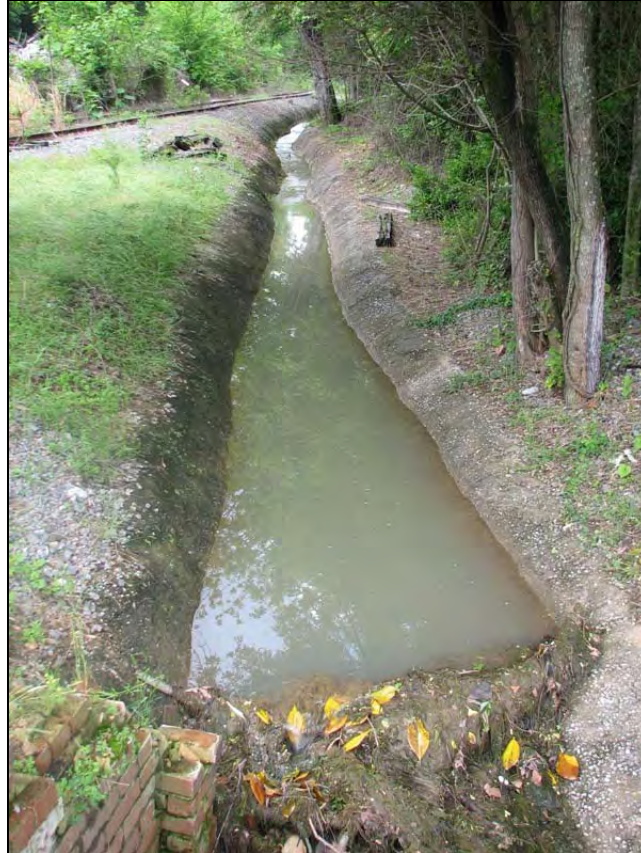
Figure 15. Drainage ditch filled with murky runoff water along the railroad tracks on the western side of Tax Parcel 167C H 002 of the Oakland Avenue and 45 th Street (Alton Park Area 3) site, Chattanooga, Hamilton County, TN. (Photo credit: Sarah Stuart Chewning and Sabrina Novak, Chattanooga-Hamilton County Health Department – 5/7/09)
