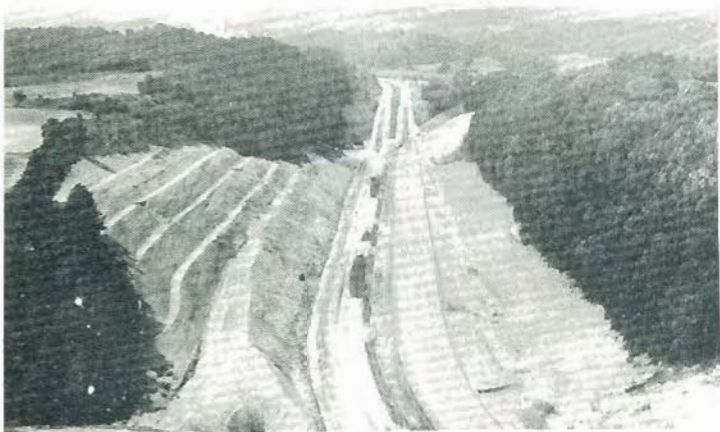
Tennessee's varying terrain presented engineers and contractors with many difficult tasks during construction of Interstates. As of July 1, 1966, some 678 million dollars in Interstate construction work has been let to contract.
