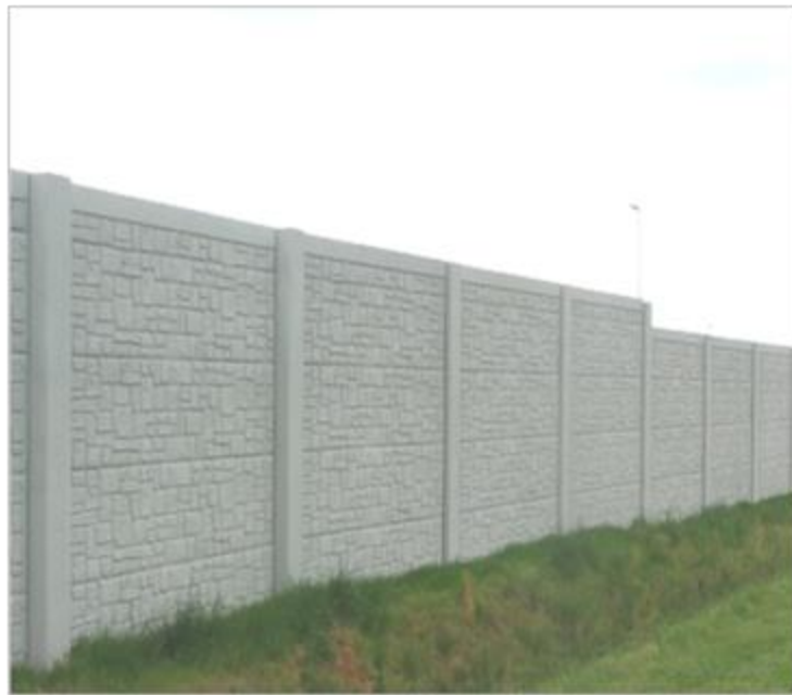
Figure 2-2: Example Noise abatement/wall (TDOT)
