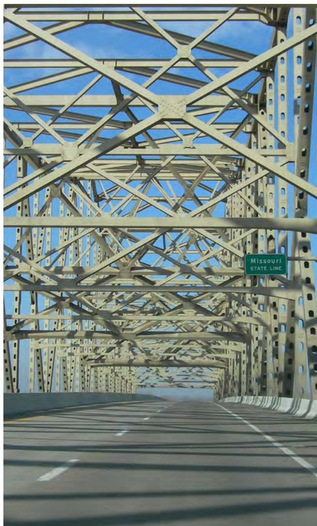
The Caruthersville Bridge carries I-155 over the Mississippi River on the west end of the study corridor.
