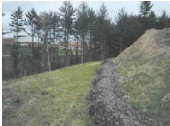
Compost Filter Berm Installed Along Contour Reference: Construction Site ESC BMPs for Iowa, (2003)
