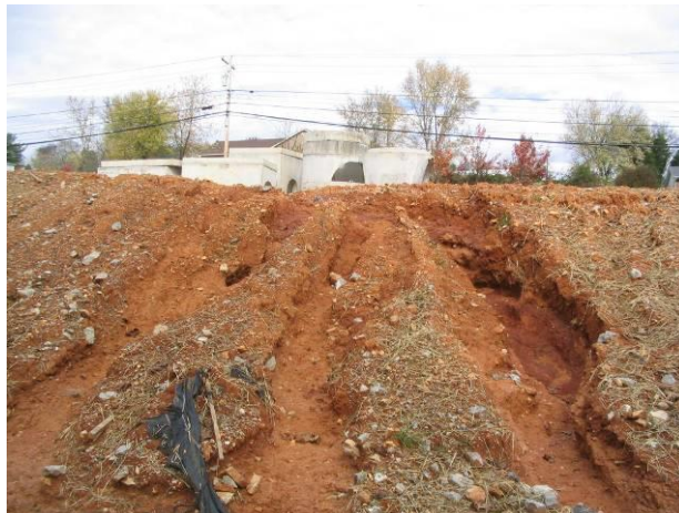
Figure 10-5 Gully Erosion on Fill Slope Location: SR-169, Knox County, TN (2004)
