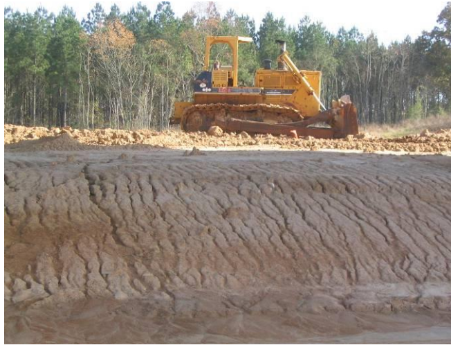
Figure 10-4 Rill Erosion on an Unprotected Cut Slope Location: SR-385, Shelby County, TN (2004)
