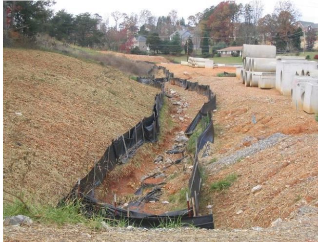
Figure 10-6 Channel Erosion Resulting from Excessive Flow and Velocity Location: SR-169, Knox County, TN (2004)
