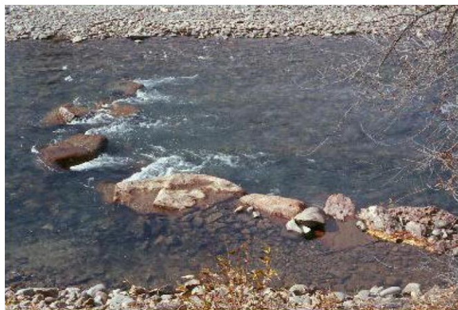
Figure 11HC-5 Typical J-Hook Rock Vane in Gravel Bed Stream Reference: U.S. EPA, Essentials of Stream Restoration (2005)
