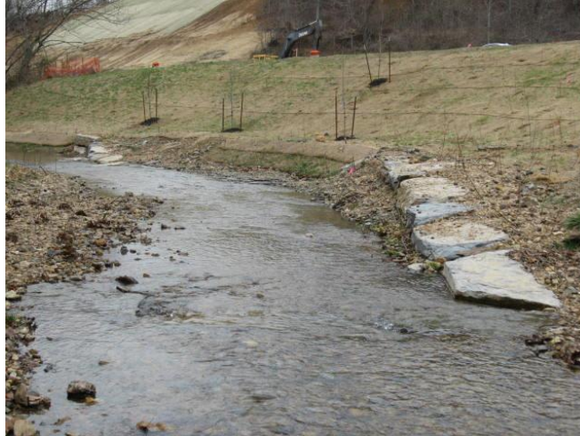
Figure 11HC-6 Typical Straight Rock Vane in a Gravel Bed Stream Location: SR-15, Furnace Branch, Wayne County, TN (2011)
