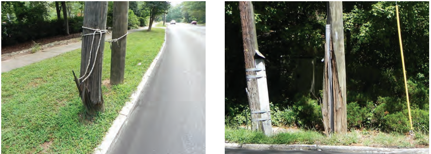
Figure 14. Examples of damaged high-risk poles (Photos: Kevin Zegeer).
