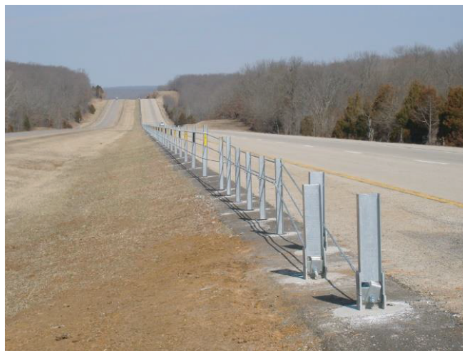
Figure 18. Example of a high-tension cable median barrier system (32).
