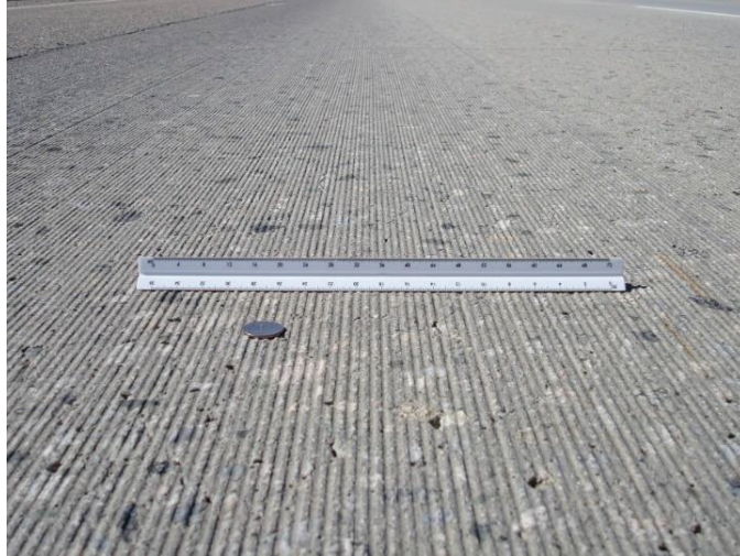
Figure 17. Example of pavement grooving (12).
