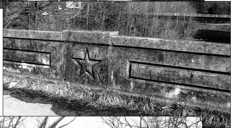
right , incised star and rectangular designs (#98, 05-NonHighway-1, the Walland Bridge east of Maryville in Blount County), built by Luten in 1918; and bottom , incised rectangular, diamond, and triangular designs; (#79, 28-01891-04.77, northwest of Pulaski in Giles County), built by Luten in 1914.
