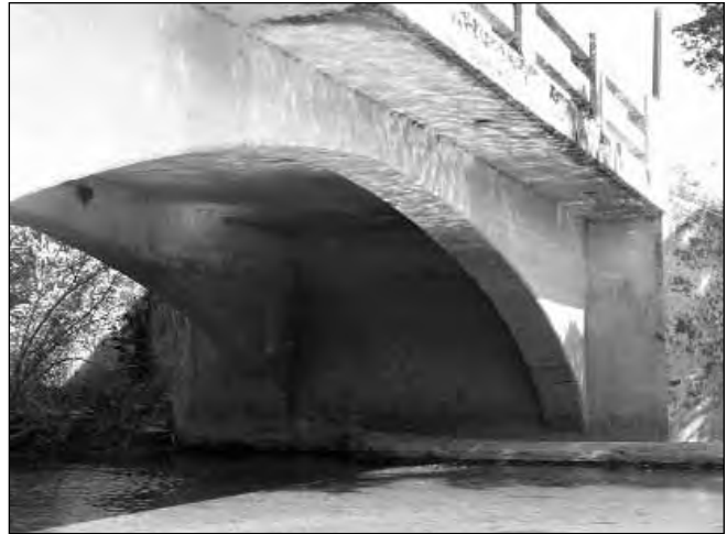
Figure IV-09: Photograph of a Filled Spandrel-Ribbed Arch Bridge in Wilson County; #124, 95-A0392-02.12, Built by Bell and Bell in 1928.
