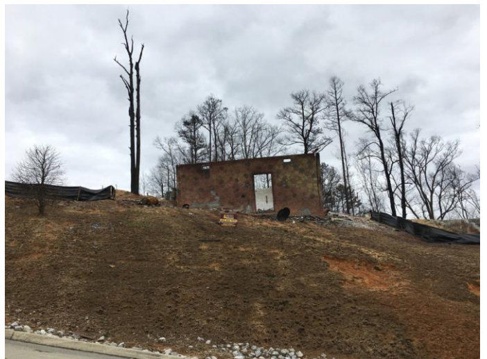
November's wildfires damaged hundreds of structures in Sevier county; sweeps uncovered over 100 likely violations.
