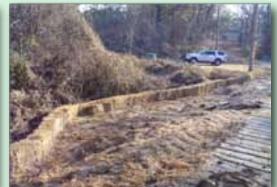
Runoff from haul road being filtered by hay bales and mats prevent rutting in Shelby County.
