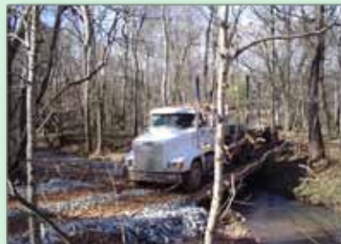
Truck crossing stream in Perry County utilizing a crossing structure and armoring.
