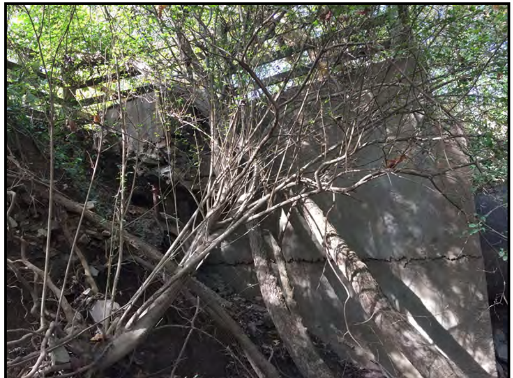
Above: Threatened sewer infrastructure in Ralston Branch
