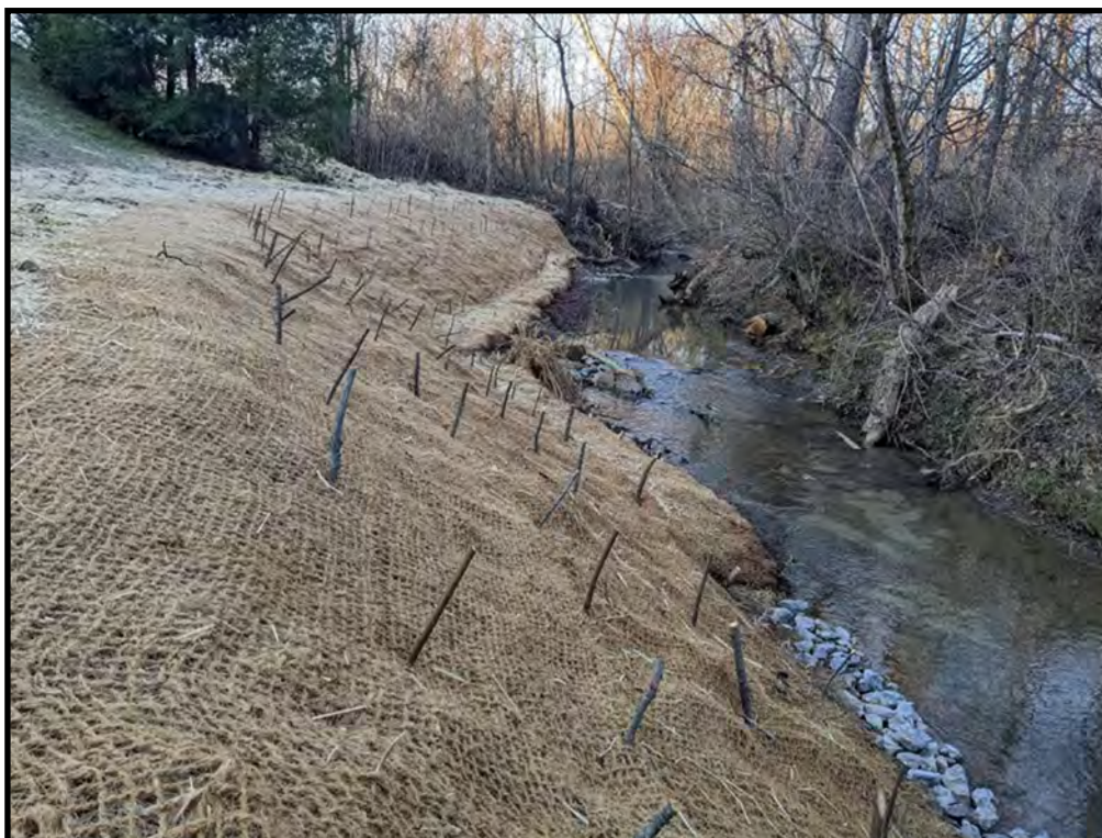
Above: After photo of Streambank restoration and stabilization on Pistol Branch in Elsborn Ridge Community
