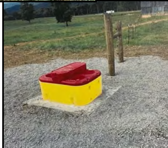
Right: Completed alternative waterer and heavy use area
