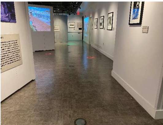
Floor outlets need to be flush with the floor surface
