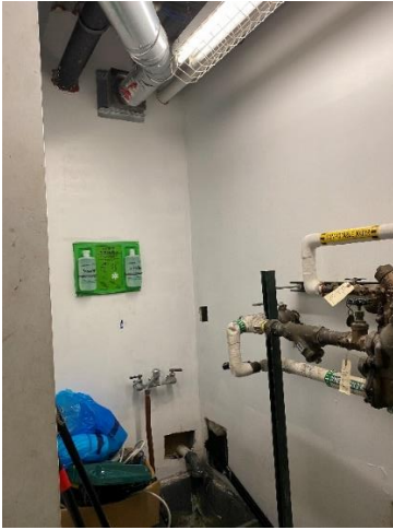
Openings need to be patched with fire rated assembly at janitor's closet
