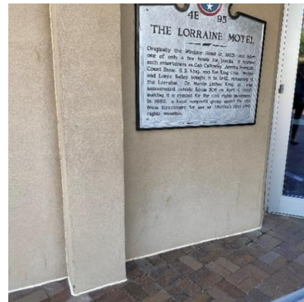
EIFS system to be repaired and repainted
