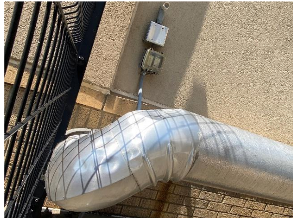
Ductwork to be repaired
