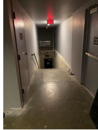
Missing handrail to be installed
