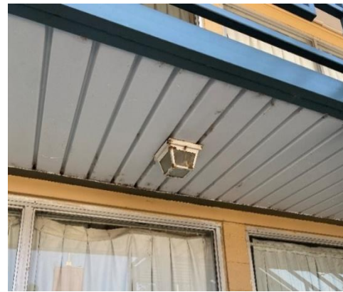
Exterior light fixtures at Lorraine Motel need replacement
