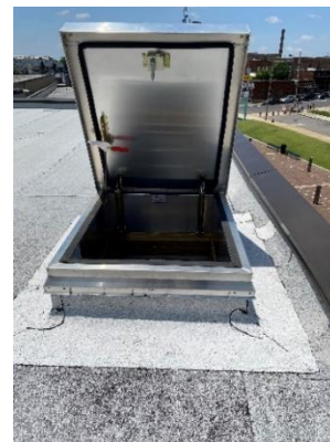
New roof hatch needs lock
