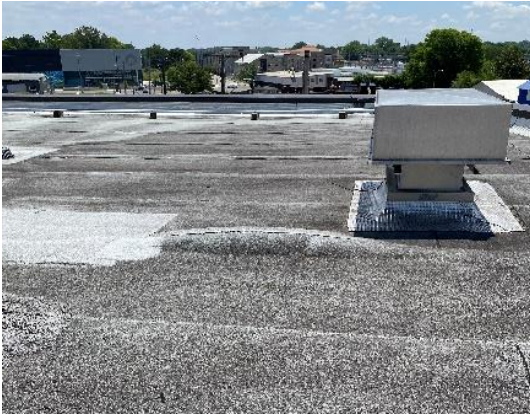
Roofing membrane that is bubbling and cracking
