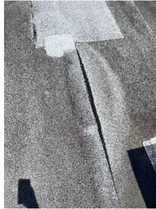
Roof membrane pulling apart at seam
