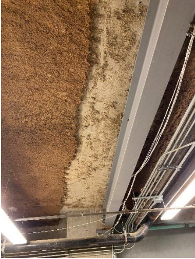
Spray insulation at basement to be reinstalled
