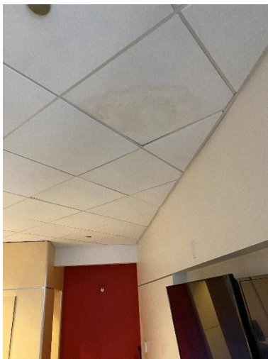
Stained ceiling tile to be replaced in Lobby
