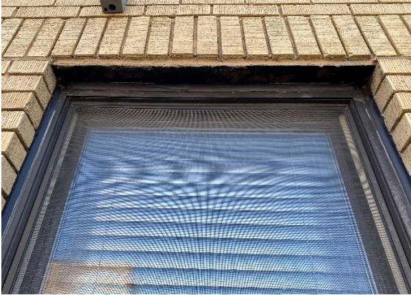
Steel lintels to be repainted
