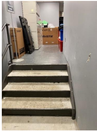
Missing handrail to be installed
