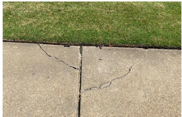
Settled sidewalk pavement to be monitored
