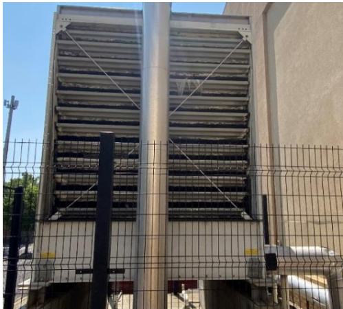
Fins of the cooling tower need to be cleaned
