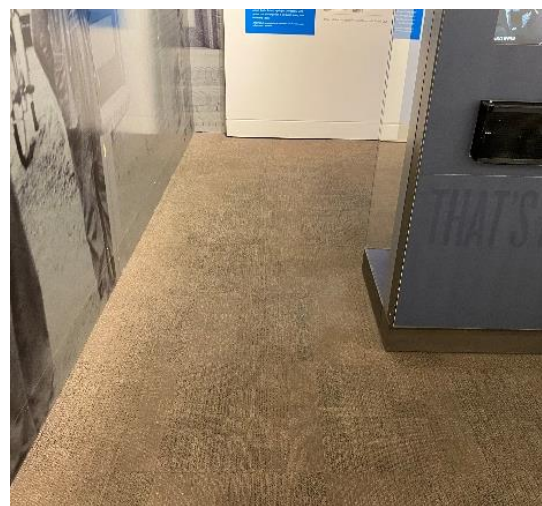
Stained and worn carpet tile to be replaced in exhibit space
