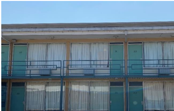
Roofing edge needs flashing at Lorraine Motel
