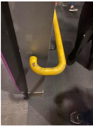
Peeling paint on handrail
