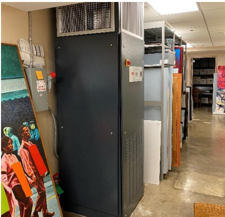
New mechanical unit in the archive room
