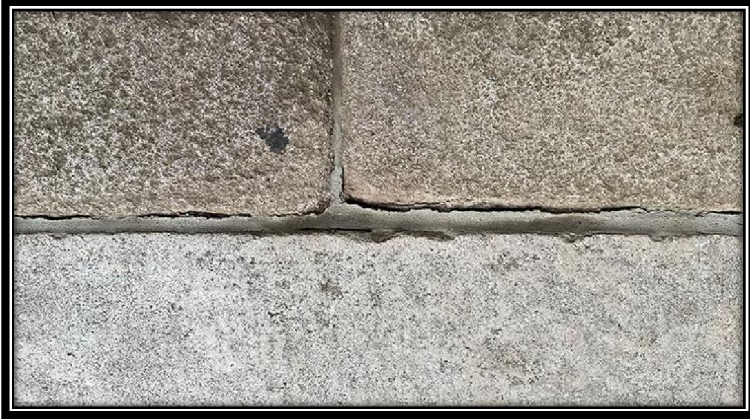
Typical sealant failure in porch floor stone joint, December 2020.
