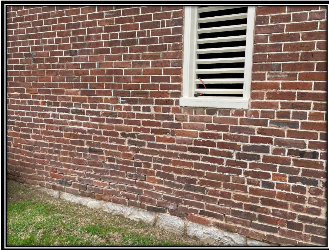
Deteriorated mortar joints on the east elevation of the Hermitage Smokehouse, December 2023.
