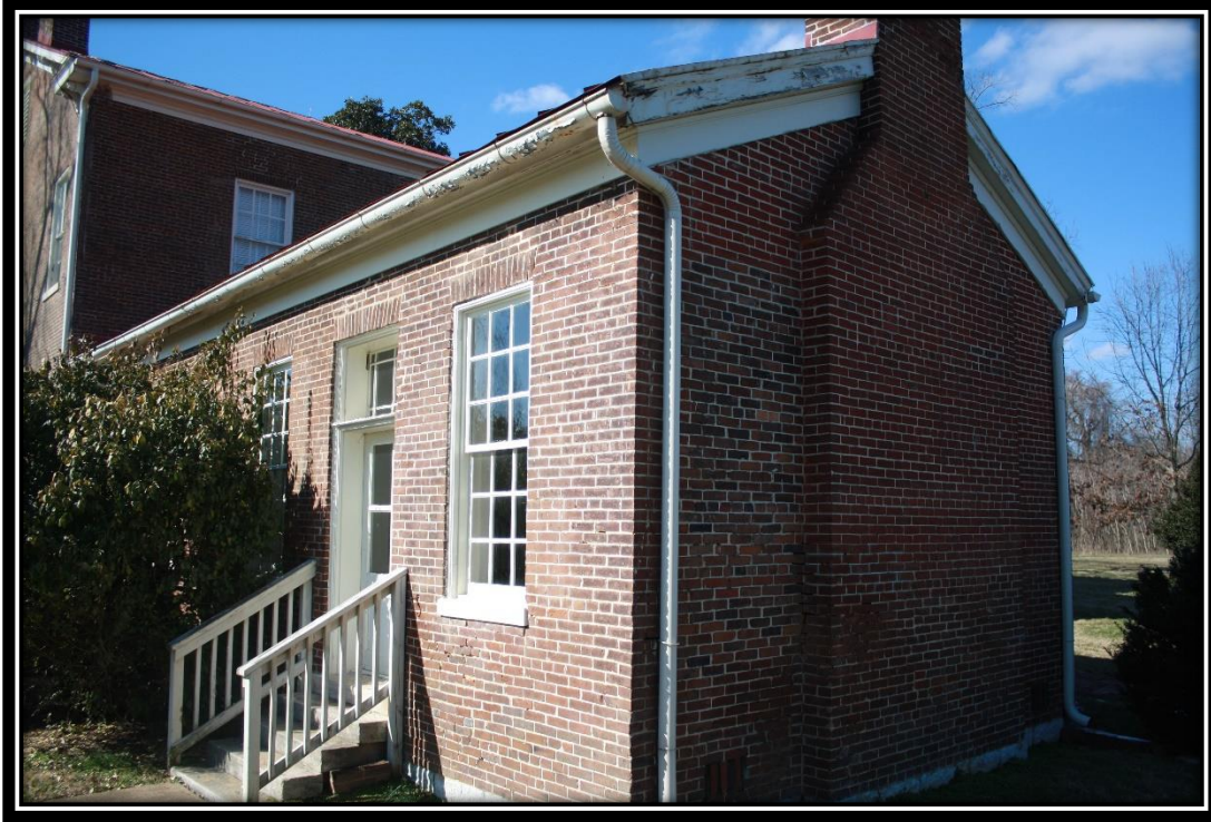
Deteriorated wood trim Tulip Grove's kitchen wing.
