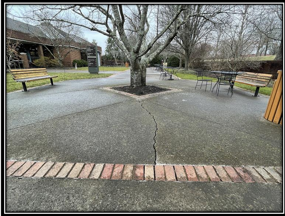
Fractured concrete slab in the Andrew Jackson Visitor Center courtyard caused by tree root upheaval, December 2021.
