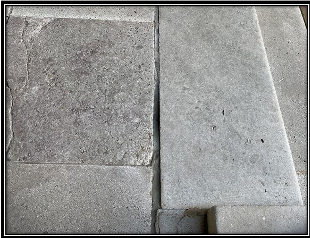
Failed joint, stone movement, and stone subsidence, December 2020.
