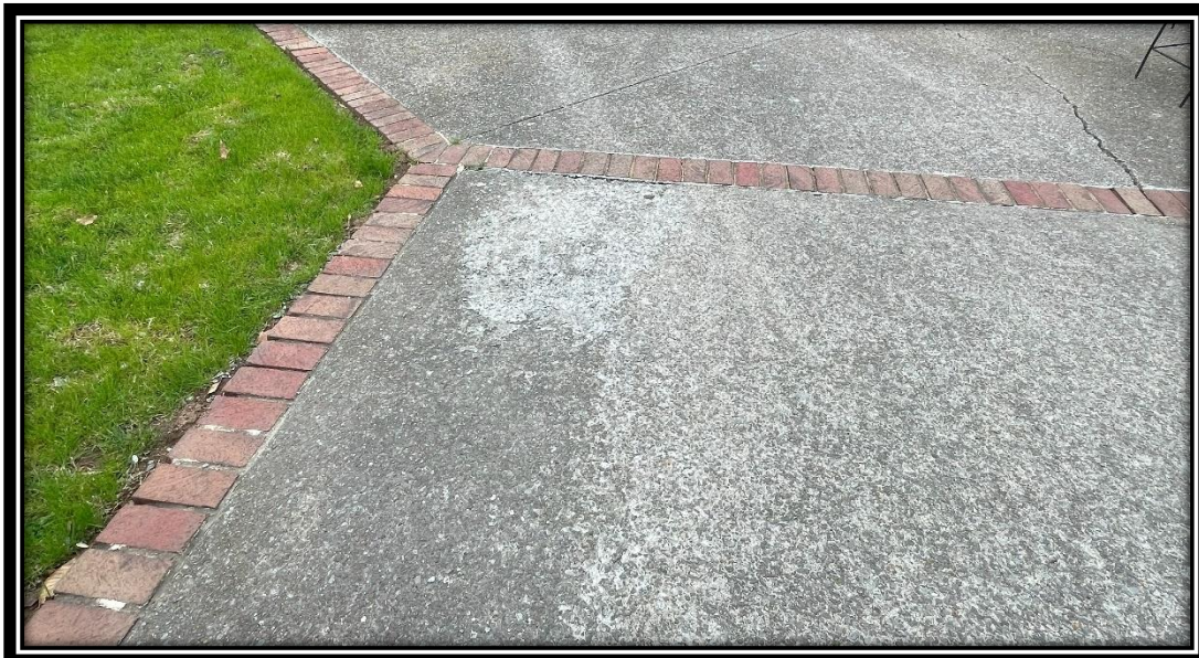
Typical concrete deterioration due to wear and salt use, December 2023.
