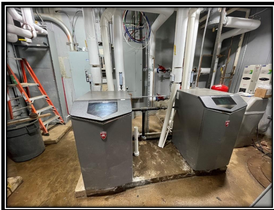
New lead-lag Lochinvar hot water boilers in the utility vault, December 2022.
