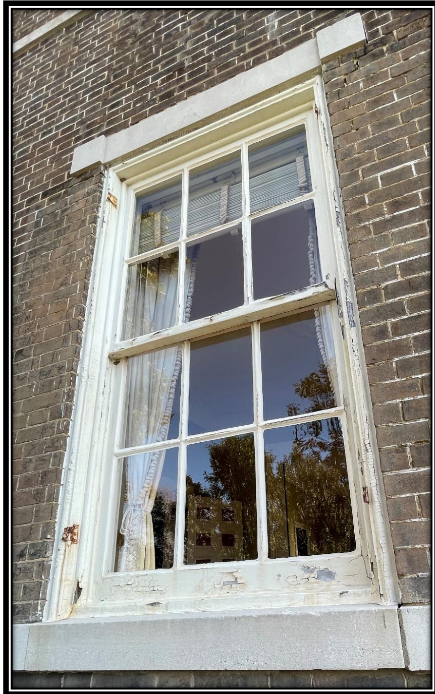
Typical window condition at Tulip Grove. All windows will be repaired, reglazed, and repainted as part of this project.
