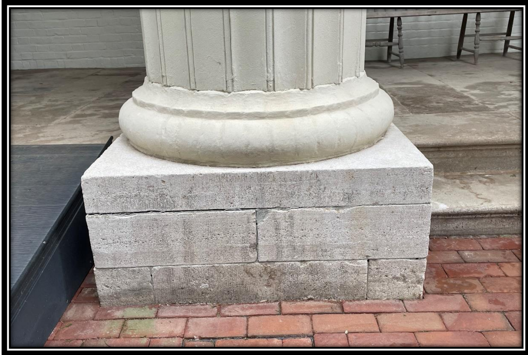
Failed sealant joints in column bases, front portico, December 2022.
