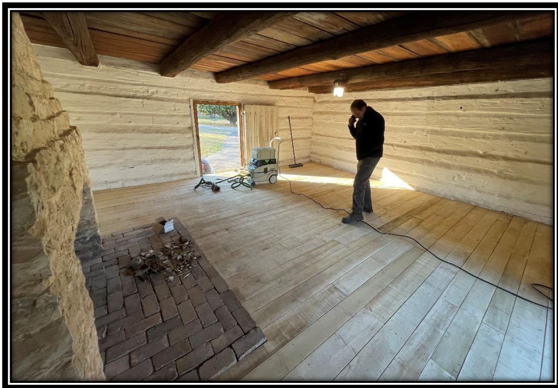
New floor installed in Alfred's Cabin, November 2022. An exhibit about enslaved housing is planned for this space.
