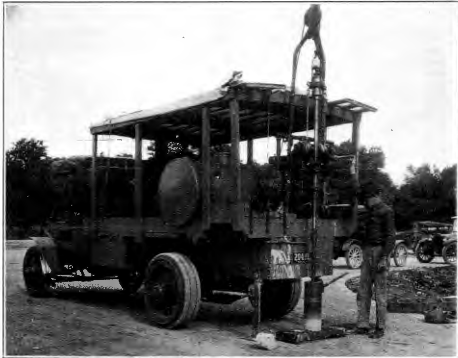
Core drill operated by Testing Division, taking cores for checking thickness and strength of pavement.
