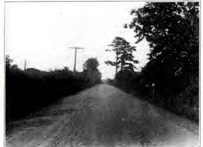
Showing surface obtained by State Maintenance on Section of Old Macadam between Knox-Loudon County Line and Concord.
