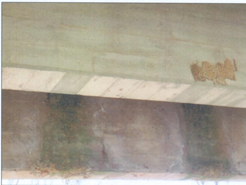
SUBSTRUCTURE CRACKING ON DOWNSTREAM SIDE OF EXISTING BRIDGE
