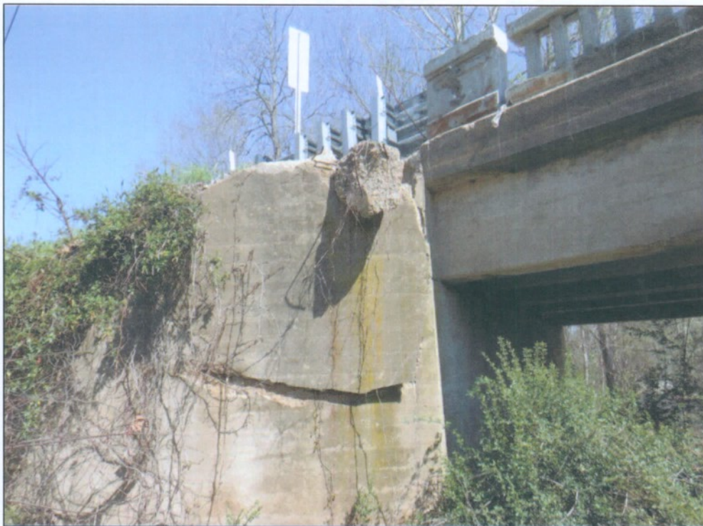
CRACKED WINGWALL ON LEFT UPSTREAM SIDE OF EXISTING BRIDGE
