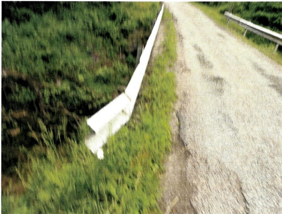
Bridge Guardrail w/ No End Terminal
