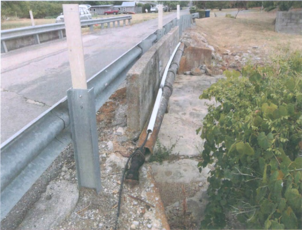
VIEW OF UTILITIES ON THE EASTBOUND SIDE OF THE BRIDGE
