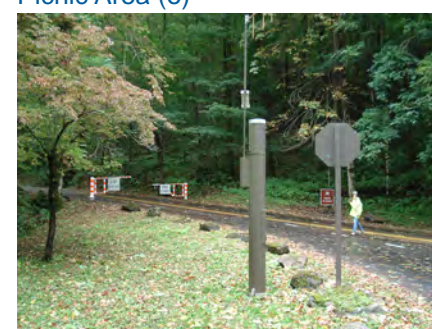
Brown, columnar communications apparatus at entrance to picnic area (-)
