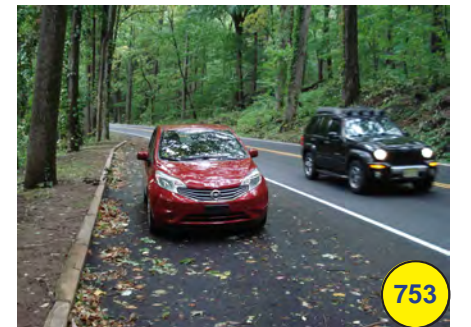
Stone curb pull off w/ muddy edge (o)
