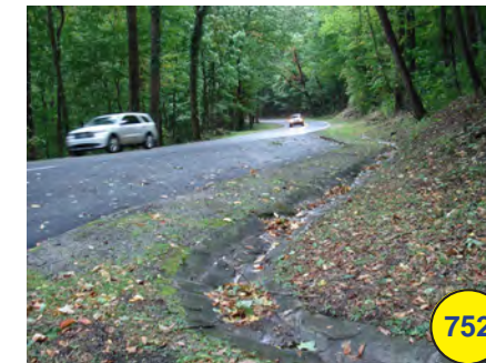
Stone and concrete swale at former Old Buckeye Trail pull off (o)
