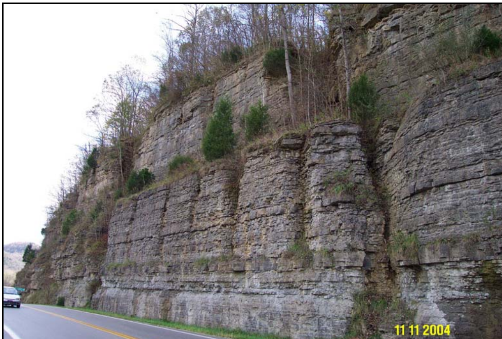
Figure 2-12: Topple and Raveling Rockfall Modes: Jackson County SR135, mile 15.5 left
