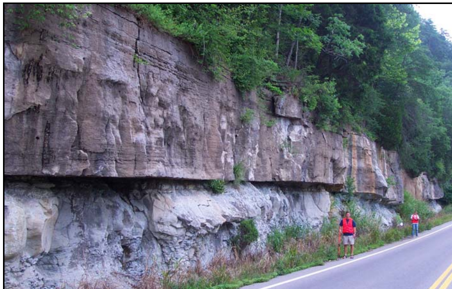
Figure 2-13: Differential Weathering and Raveling Rockfall Modes: Cheatham County SR070, mile 4.6 left
