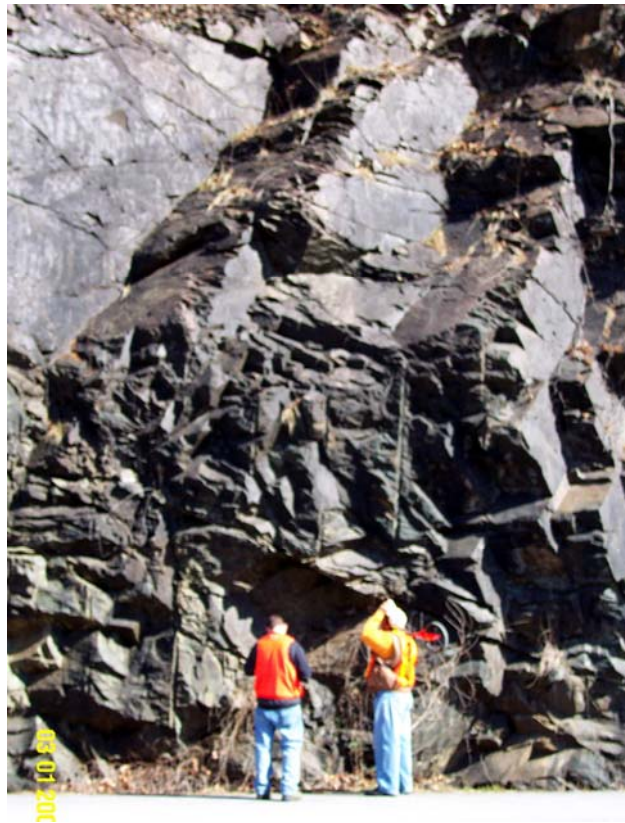
Figure 2-10: Wedge Rockfall Mode: Carter County SR-37, mile 14.1 right
