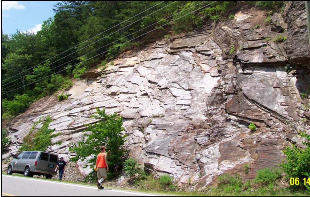
Figure 2-9: Planar Rockfall Mode: Blount County SR115, mile 14.6 right
