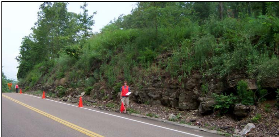
Figure 2-16: Raveling Rockfall Mode: Decatur County SR100, mile 9.95 right
