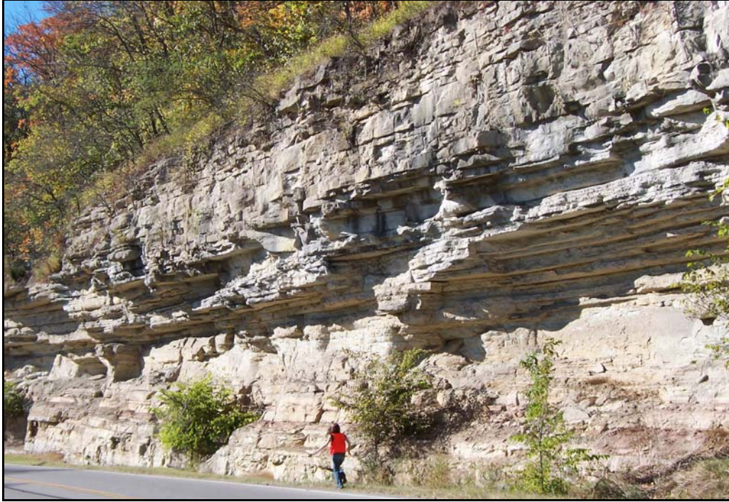
Figure 2-14: Differential Weathering and Toppling Rockfall Modes: Davidson County SR001, mile 2.4 left
