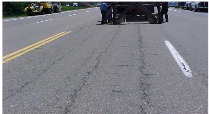
Extensive cracking from oxidized pavement
