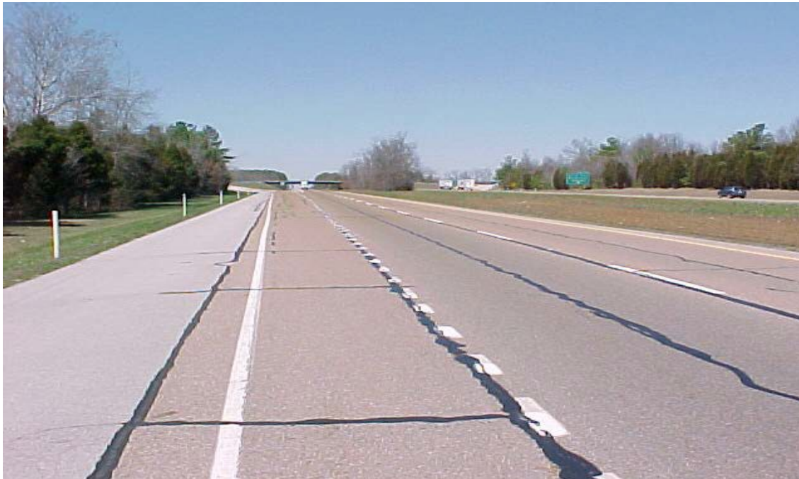
Quantity of crack seal is excellent; however, longitudinal crack seal is too heavy.
