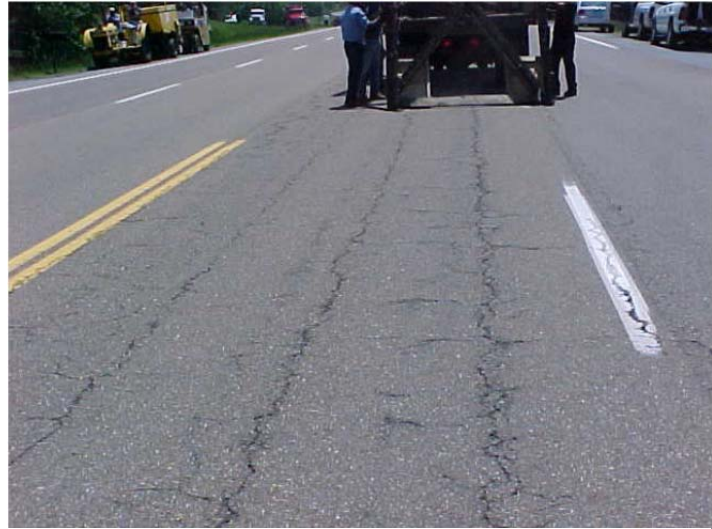
Extensive cracking from oxidized pavement, no structural damage
