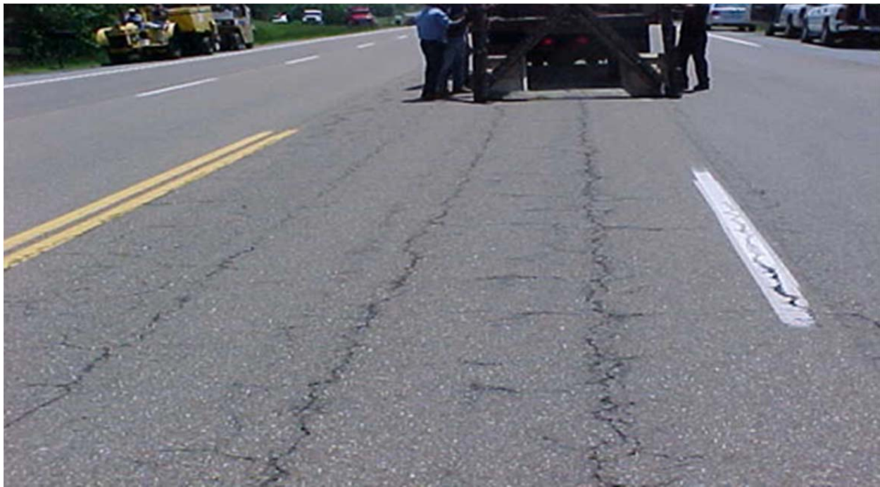
Extensive cracking from oxidation, no structural damage
