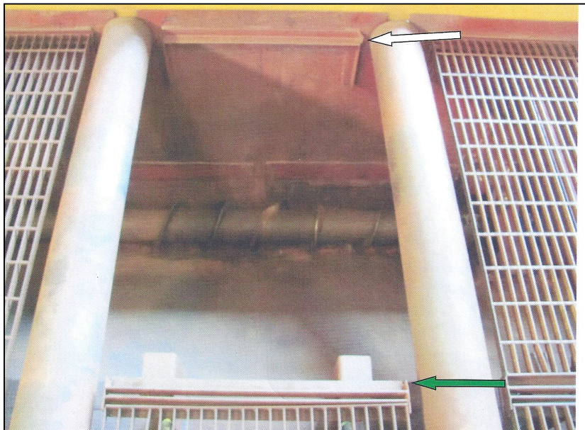
Opening that the victim fell through and auger he fell onto
