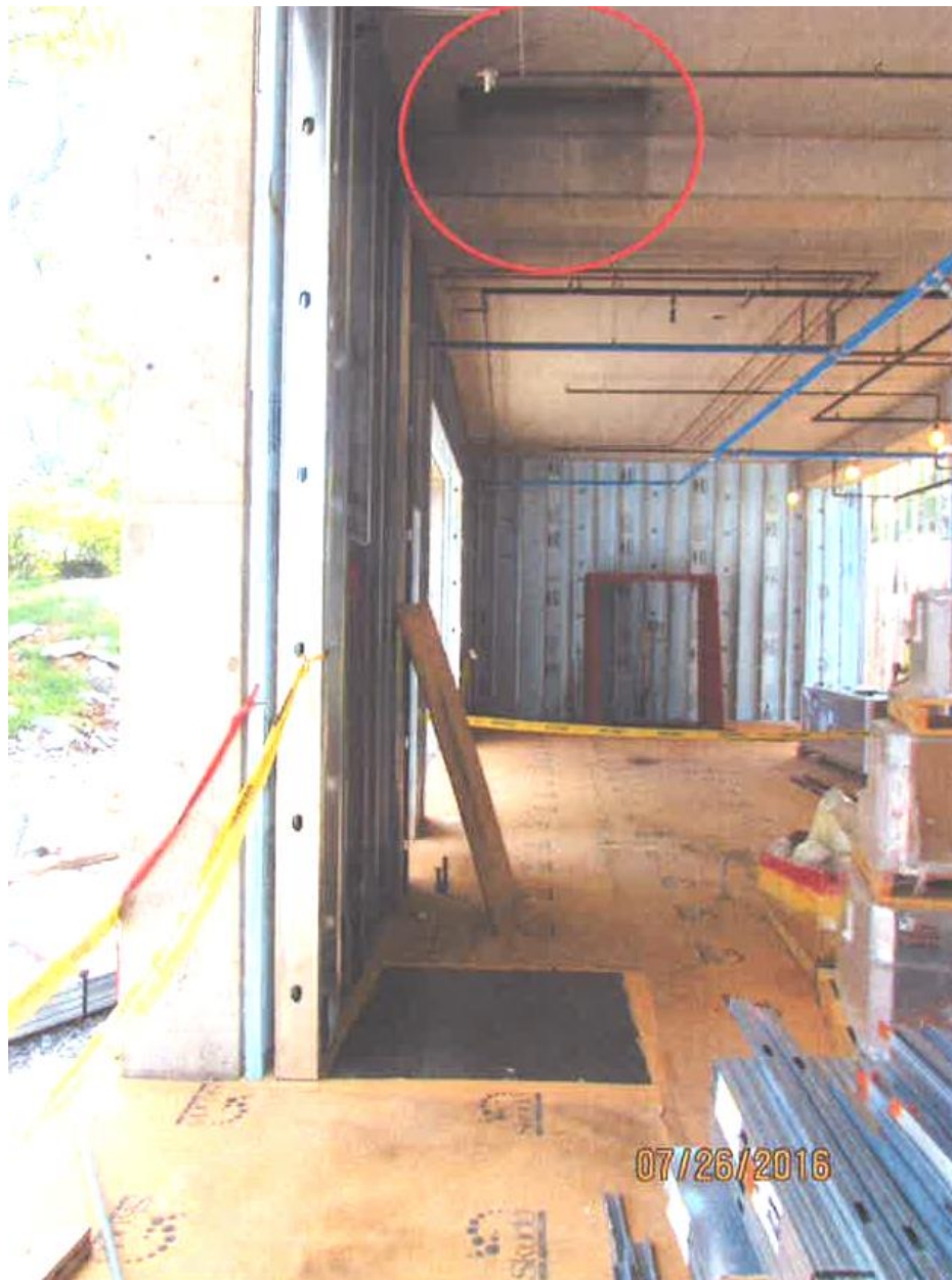
Photo 2 of 2 – The red circle indicates where the victim fell through the floor opening cover into the basement below.
