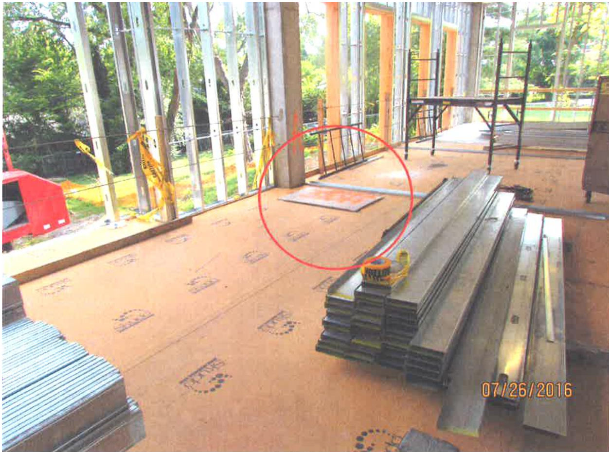
Photo 1 of 2 – The red circle indicates where the floor opening was located near the windows.
