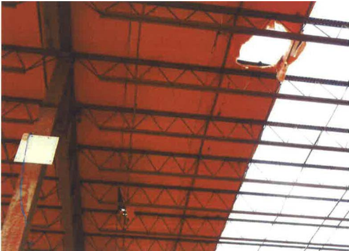
Photo 1 of 1 – Location of where the victim fell through the insulation on the roof.
