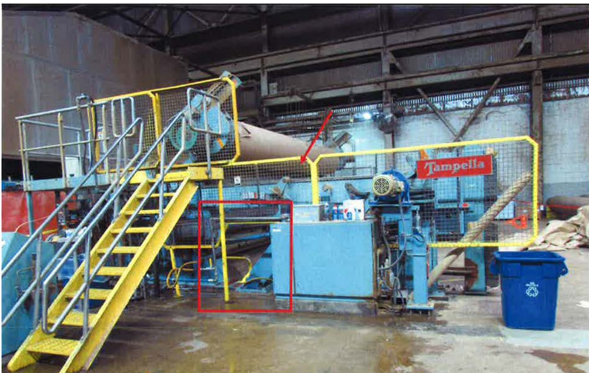
Photo 2 of 2 – The victim went under the guard designated by the red square, and was crushed by the secondary arm and the frame of the Tampella winding machine. There were guards designated by the red arrow in place on each side of the machine, but they did not keep employees from going under them.
