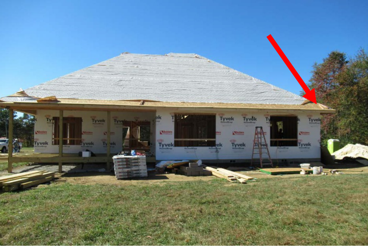
19 fall from roof--Inspection #1438651 Lorenzo Garcia
