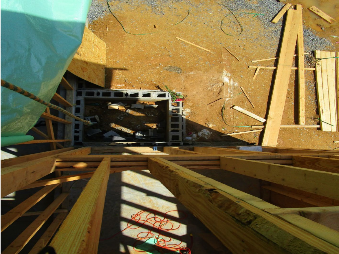
26 Fall from second floor—Insp#1488550 Ruben Escorza-Dimas
