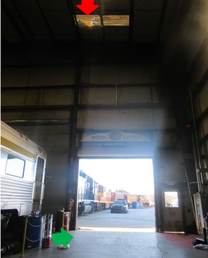
Fall through skylight —Insp # 1641715 Tennessee Valley Railroad
