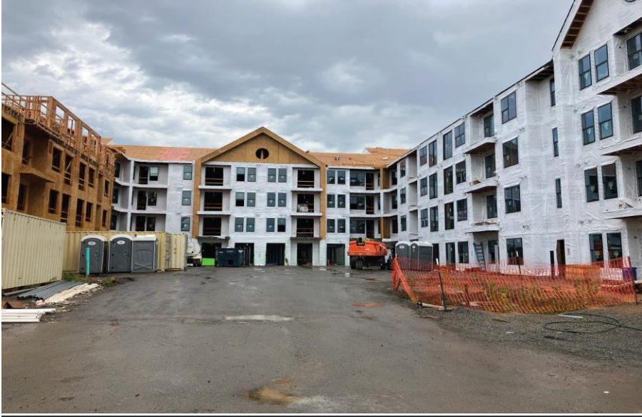
Fall from roof—Insp # 1700418 Juan Montiel
