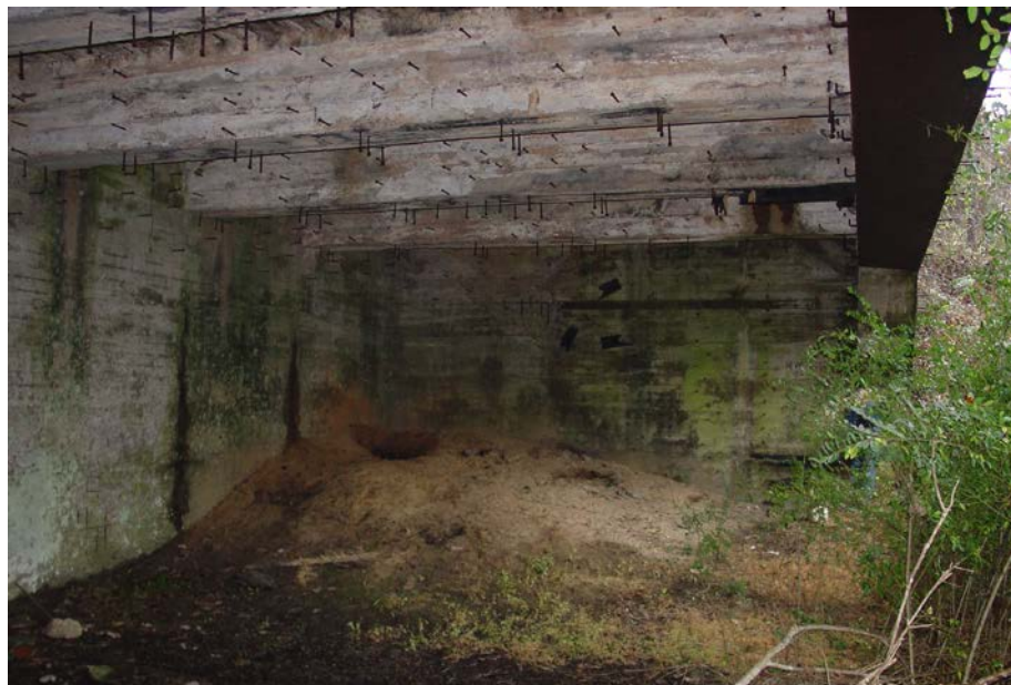
Figure 14. Interior of target butt at William Northern Field (TDOA WWII image file, photo #S094).
