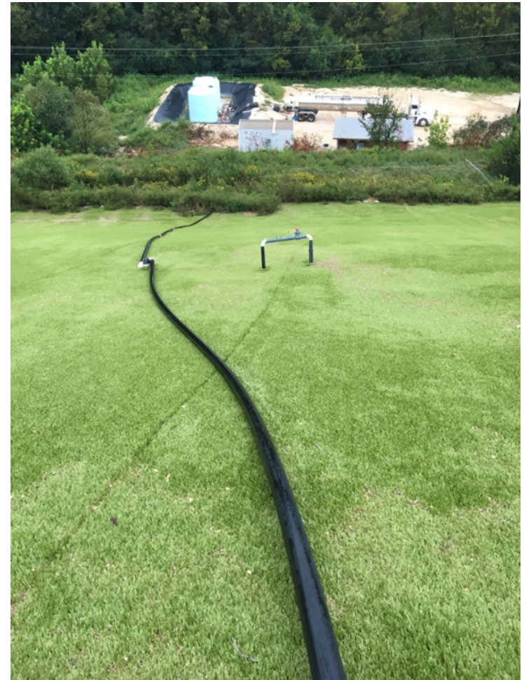
Header Line to Gas Management Bldg.
