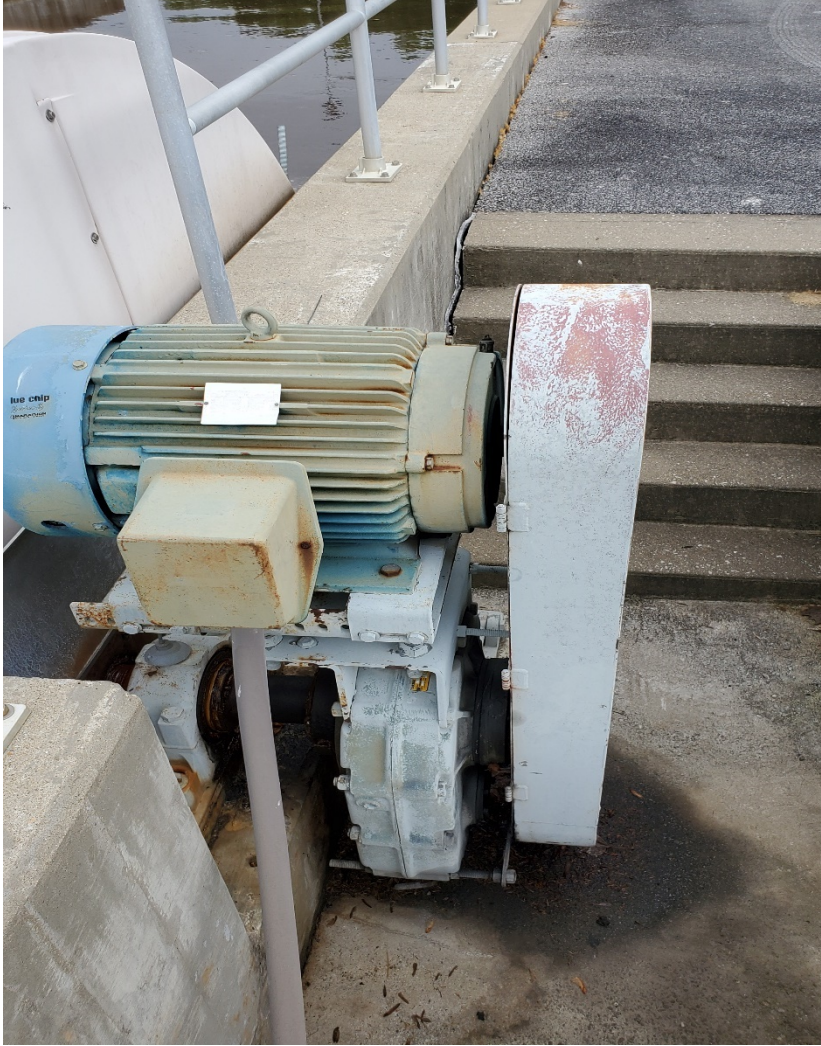
Aeration rotors (4 @ 50 HP each; fixed speed, no VFD, no soft-start)
