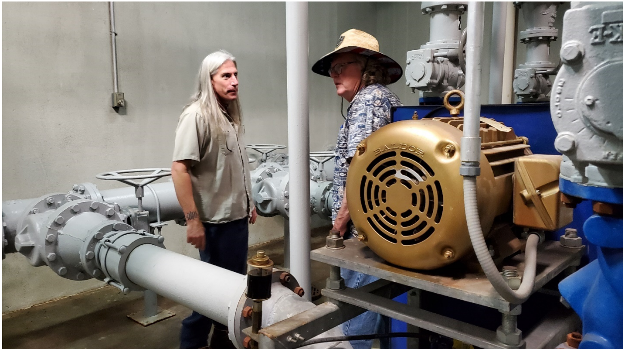
Grant Weaver of CleanWaterOps and Harriman WWTP Chief Plant Operator Ray Freeman discuss the equipment and RAS and WAS procedures.
