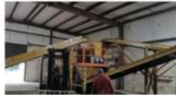
Granutech primary shredding line
