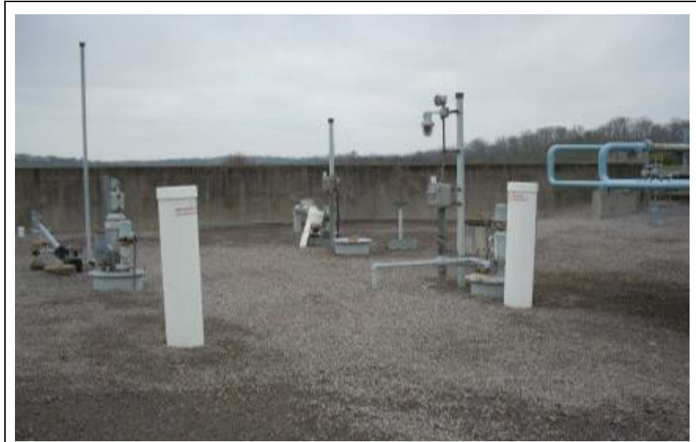
Example Tank Configuration at a Bulk Terminal
