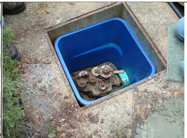
Uncontained sump using a plastic container to keep backfill from caving in on pump head. This would not meet present installation standards.
