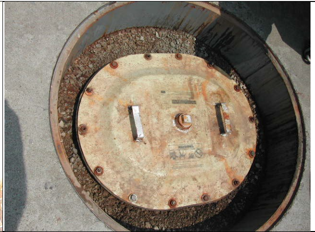
Oval-shaped sump on fiberglass reinforced plastic (FRP) tank top
