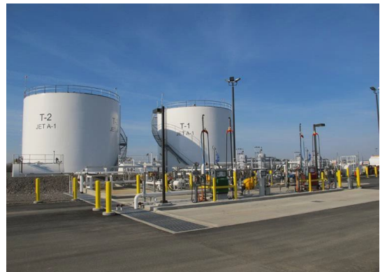
Example Fuel Farm with USTs and ASTs
