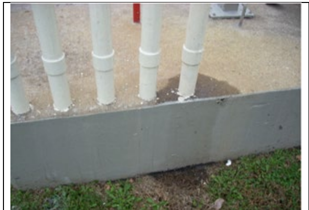
An Overfilled Tank May Cause a Release from the Vent Pipe
