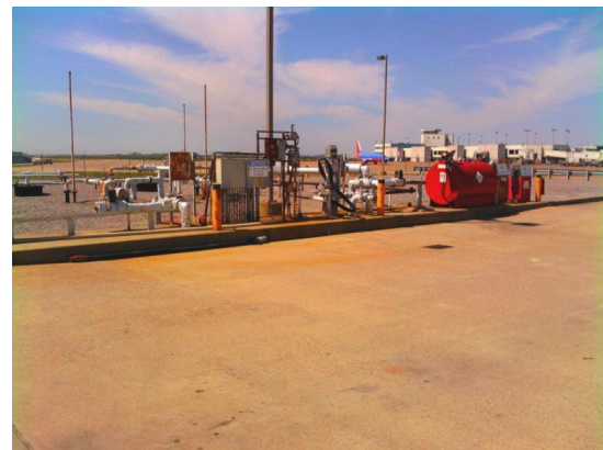
Curbside Fuel Loading/Offloading
