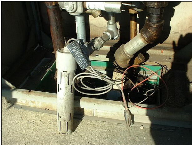
Shallow Under Dispenser Containment Sump with Sensor
