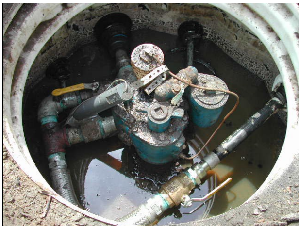
Water and product in sump and sensor have been moved out of position and cannot properly detect liquids in sump
