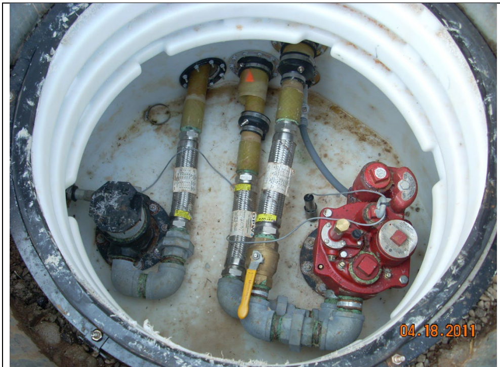
Pressurized emergency generator system equipped with an interstitial sensor.
