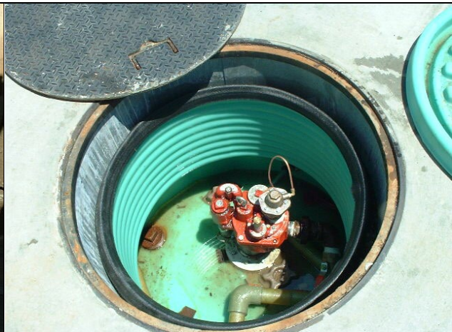
Typical STP Sump Showing Sump Lid and Cover
