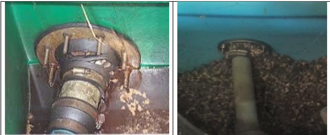
The photos above show damaged penetration fittings allowing gravel to backfill to enter the sump. The sump is no longer liquid-tight.
