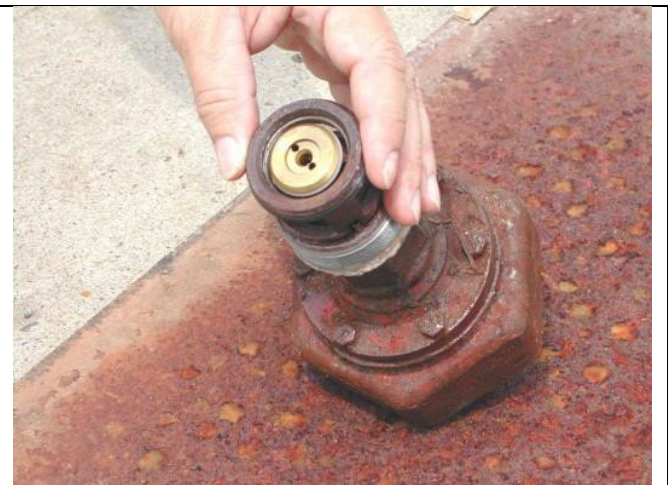
Tampering with a leak detection device is a CRIMINAL OFFENSE
