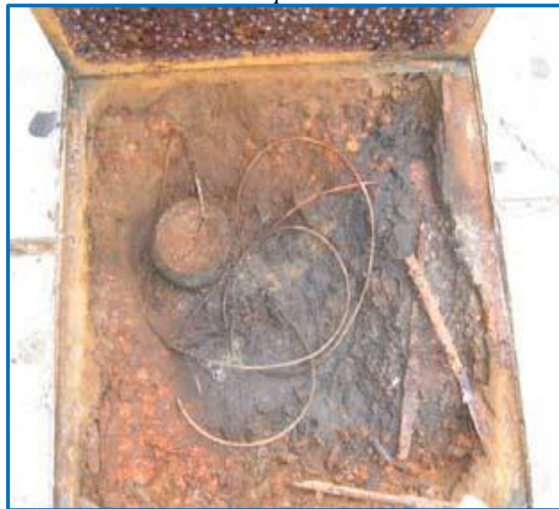
Corroded Incompatible ATG Probe
