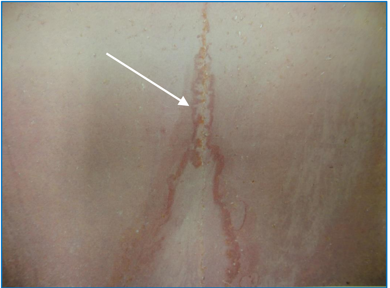
UST 89 Octane internal view: crack
