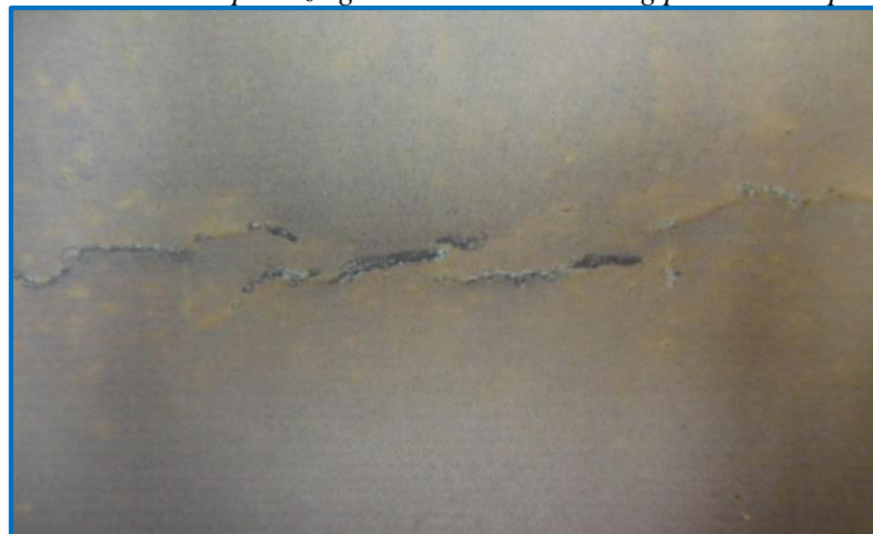
92 Octane UST – deep crazing/crack observed during pre-blast inspection
