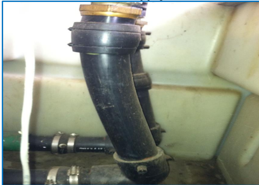
Supporting Pictures: Bent UPP piping
