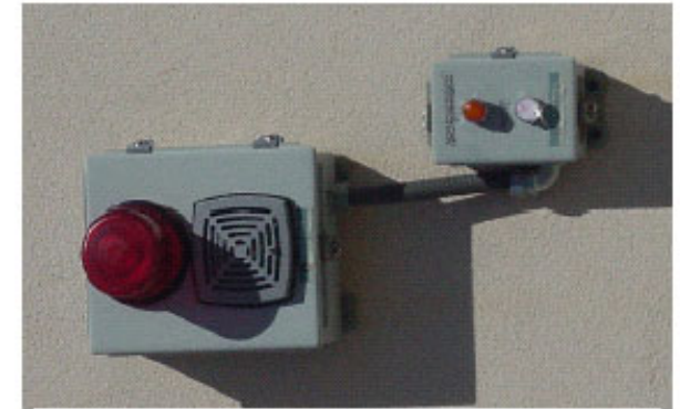
Sample Overfill Alarm
