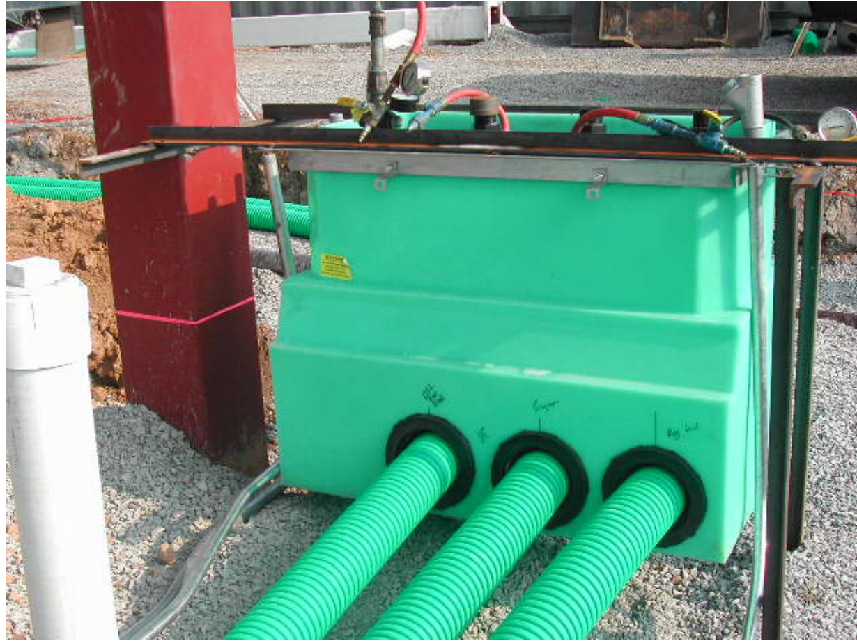
Dispenser containment sumps with secondarily contained piping
