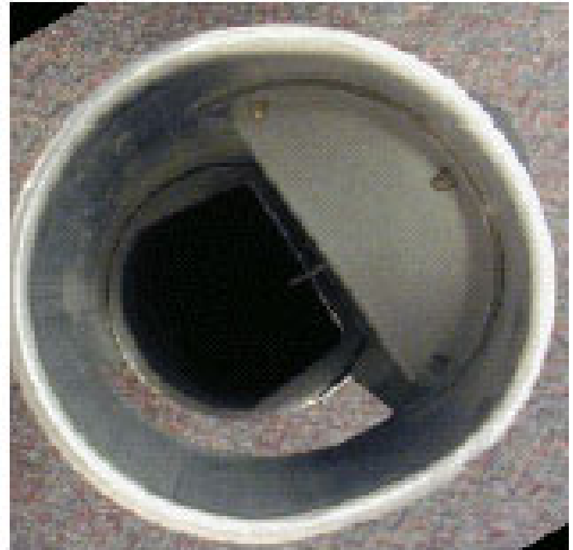
Looking Through The End Of Automatic Shutoff Device
