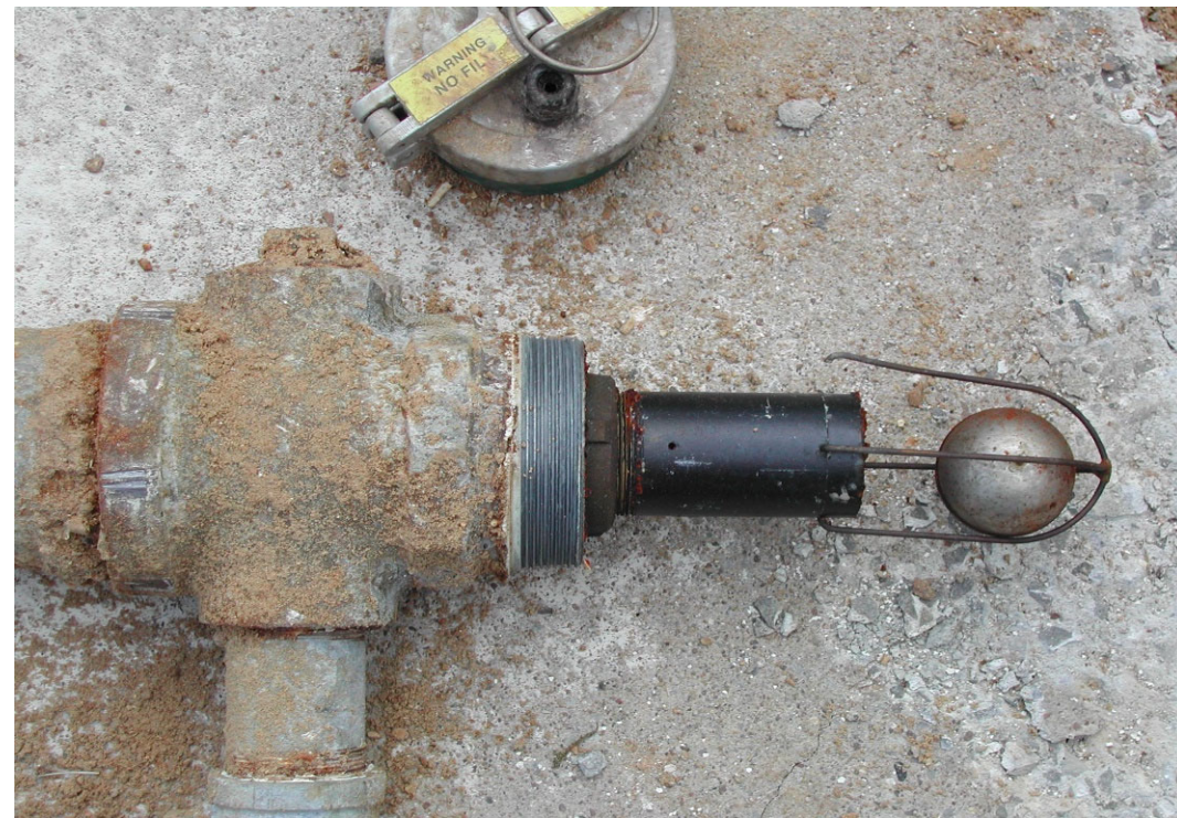
Wire restraining cage is loose
