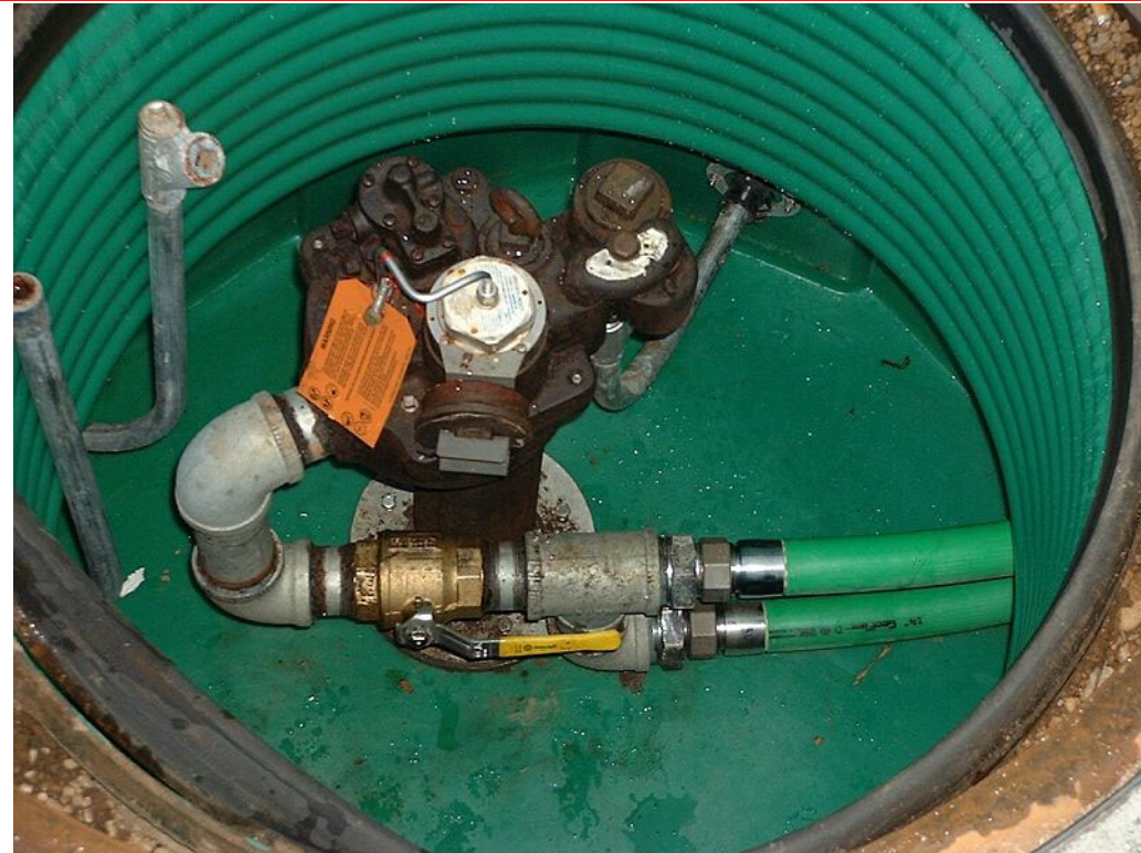
Flexible plastic piping
