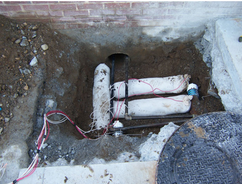
Bag anodes attached to metal piping
