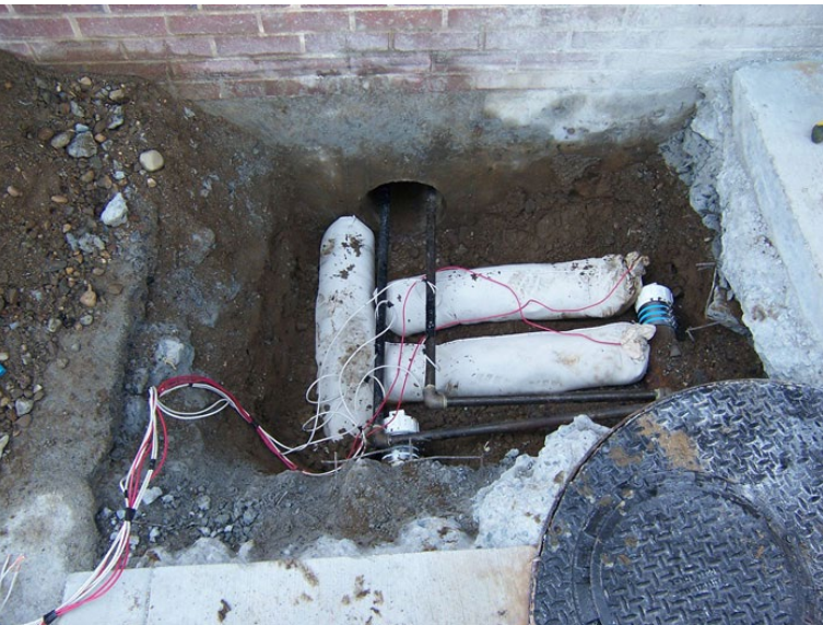
Bag anodes attached to metal piping
