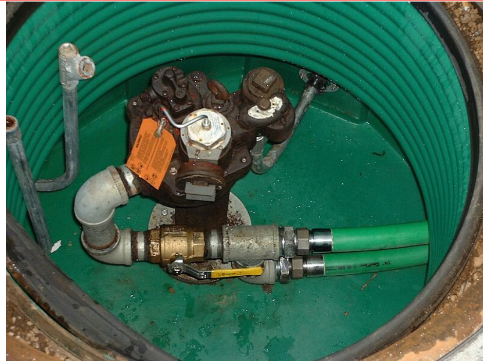
Flexible plastic piping
