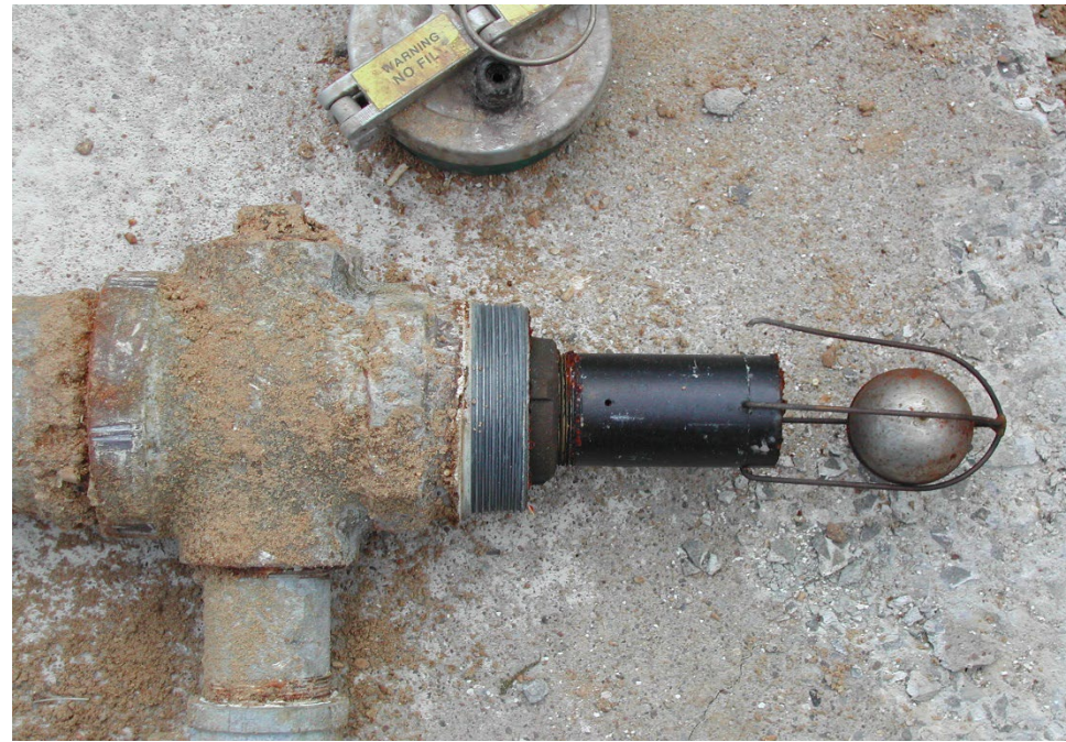
Wire restraining cage is loose
