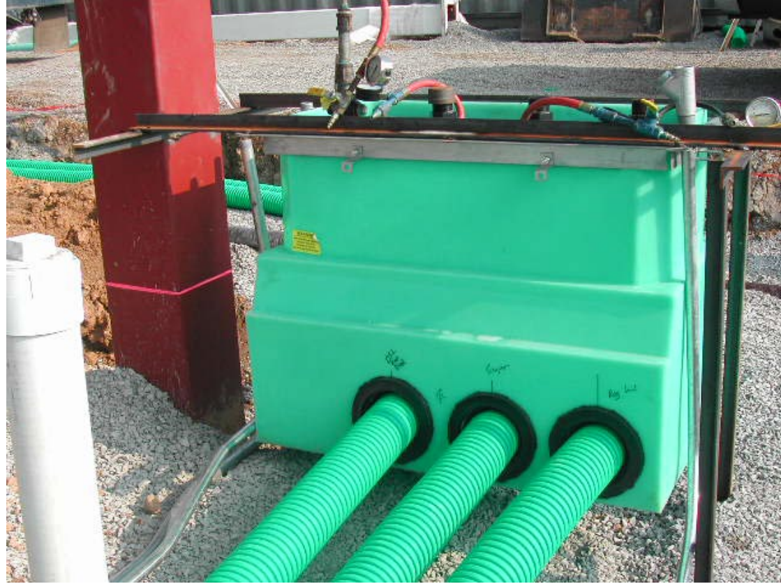
Dispenser containment sumps with secondarily contained piping
