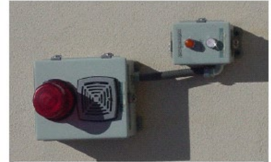
Sample Overfill Alarm
