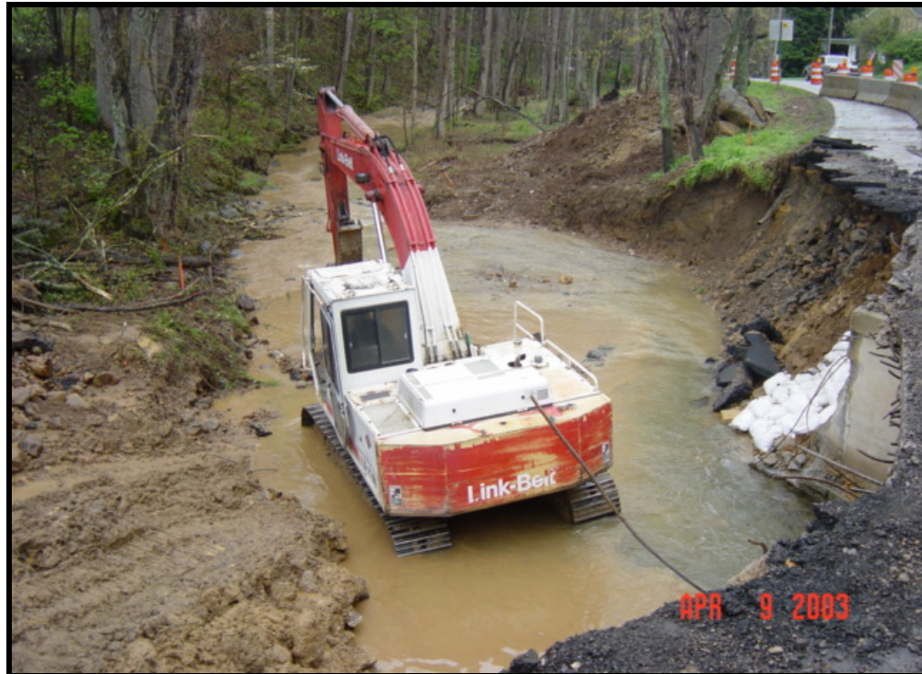
Construction activities that utilize improper techniques such as the placement of heavy equipment instream leads to erosion, loss of habitat, and sedimentation. Photo provided by Andrew Tolley, Johnson City OFFICE.
