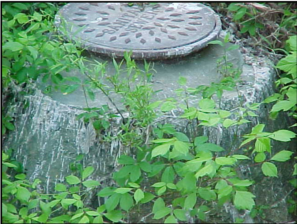
Sewer overflows allow untreated sewage to enter waterways.
