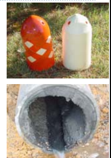
Pipe with sludge before cleaning
